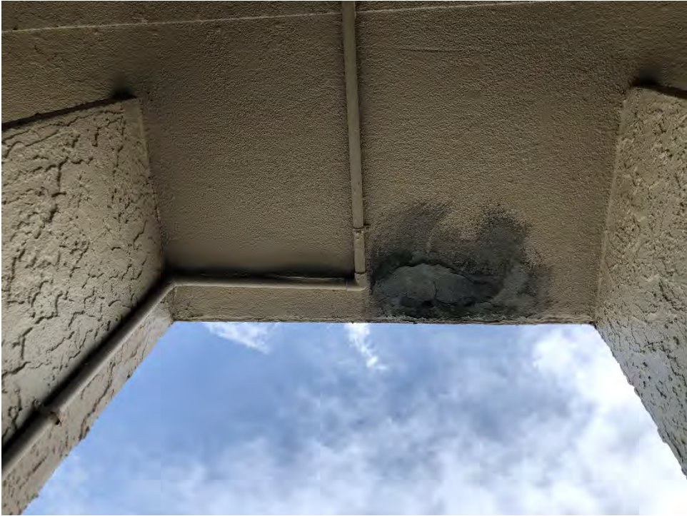
Figure D- 25 – Concrete Spall
