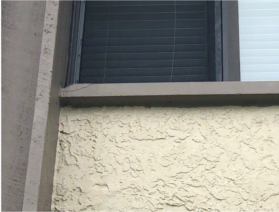
Figure E- 45 – Windowsill Spall (Unit 305)
