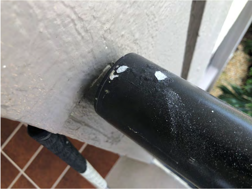
Figure B- 9 – Typical Guardrail Peeling Paint/Oxidization
