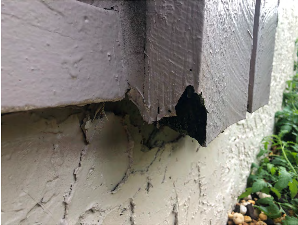
Figure E- 67 – Typical Wood Trim Rot
