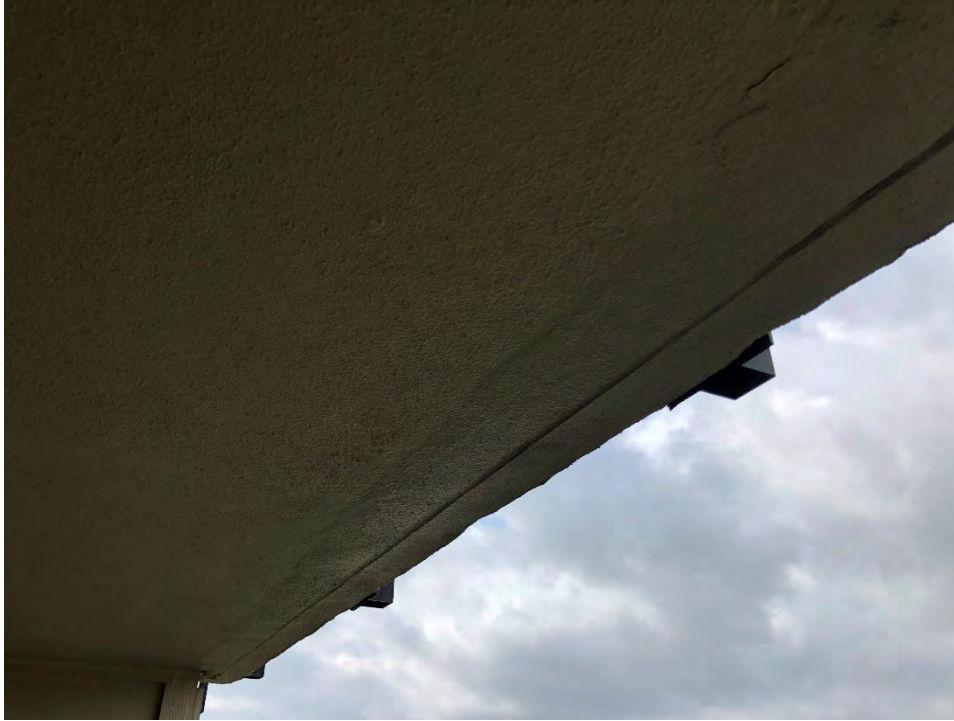
Figure A- 15 – Unit 220 Delaminated Exterior Ceiling Stucco Finishes
