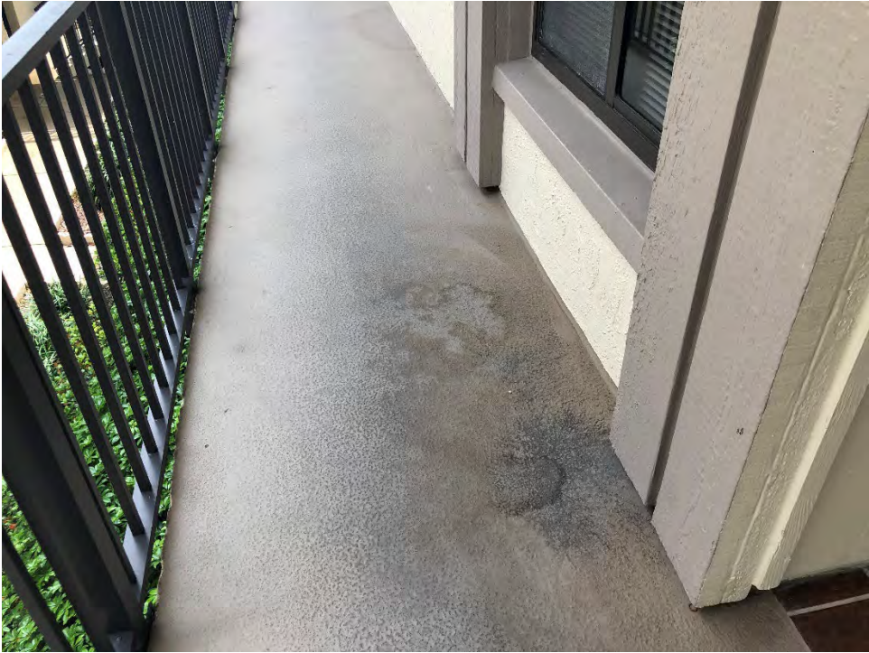
Figure B- 13 – Ponding Water
