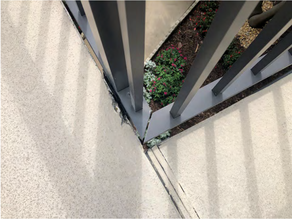
Figure B- 17 – Loose Bottom Rail Connection
