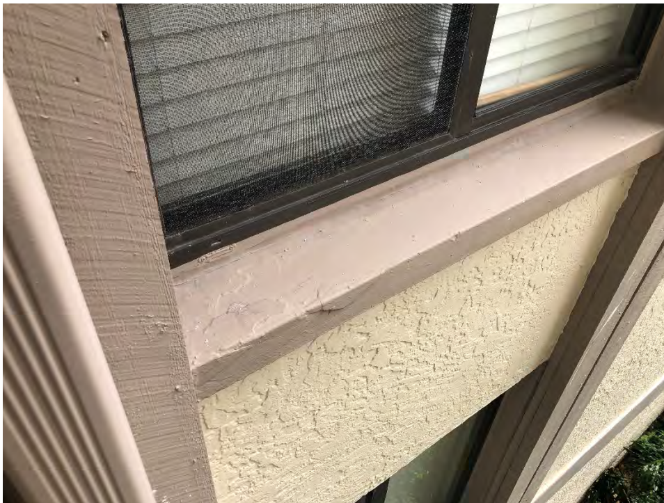
Figure E- 40 – Windowsill Spall (Unit 304)
