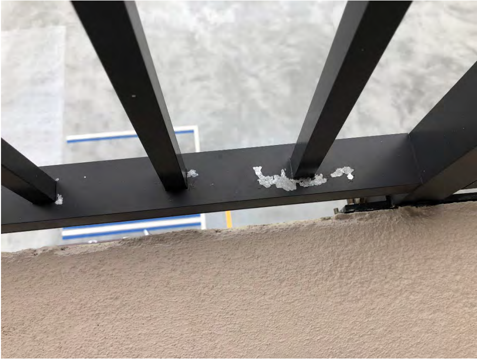
Figure A- 5 – Typical Tower Guardrail Peeling Paint/Oxidization
