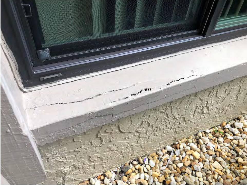
Figure E- 35 – Windowsill Spall (Unit 104)
