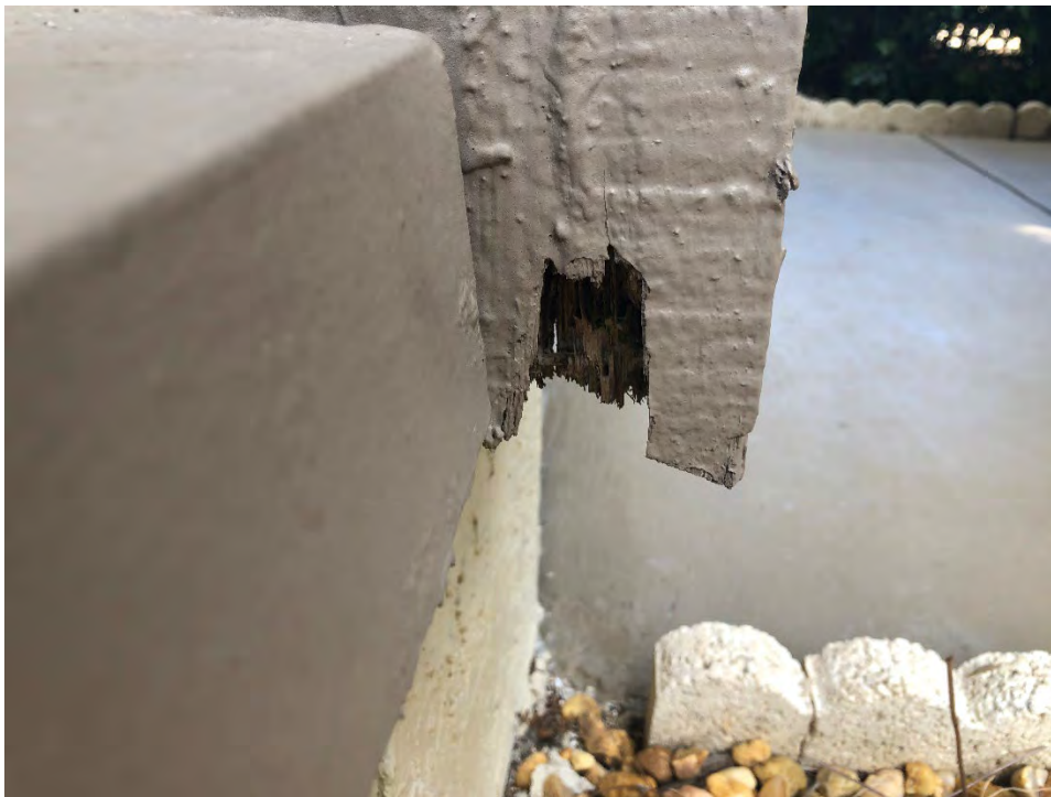
Figure E- 66 – Typical Wood Trim Rot
