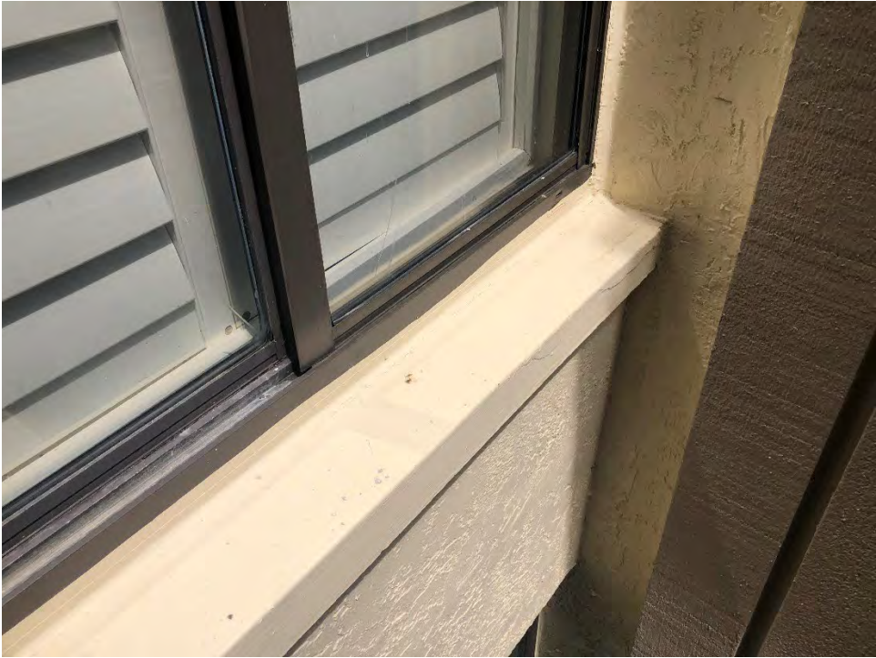
Figure E- 37 – Windowsill Spall (Unit 203)
