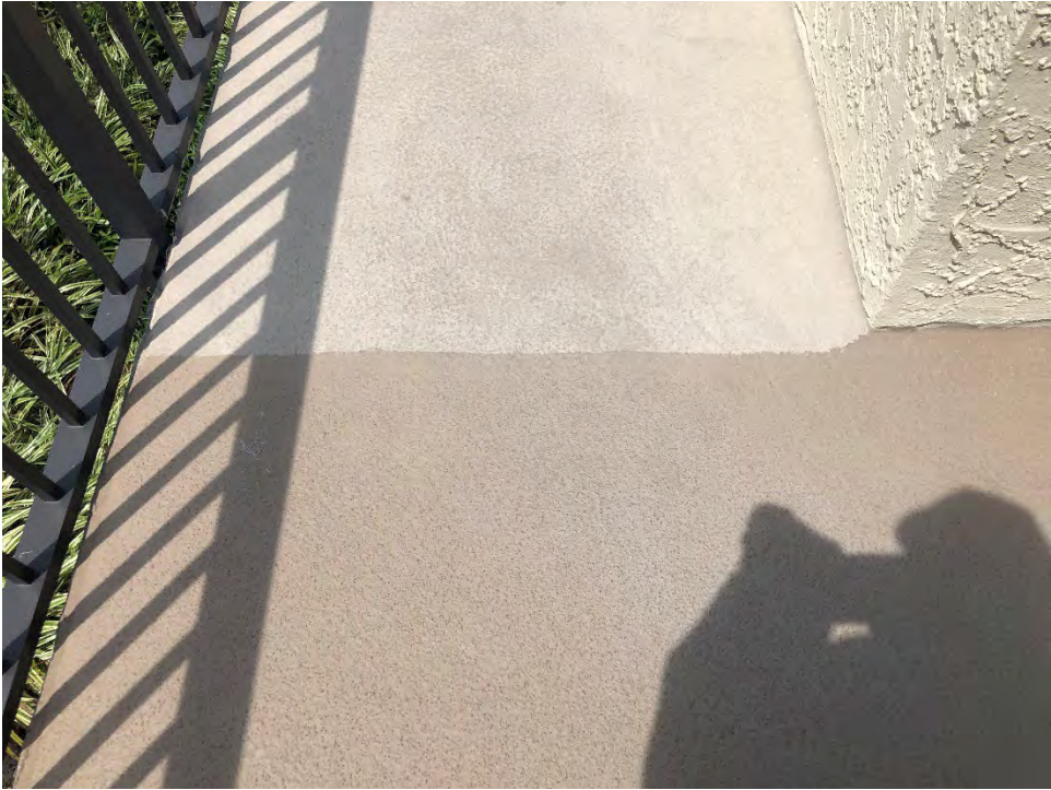
Figure B- 11 – Deteriorated Waterproofing Membrane Top Coating
