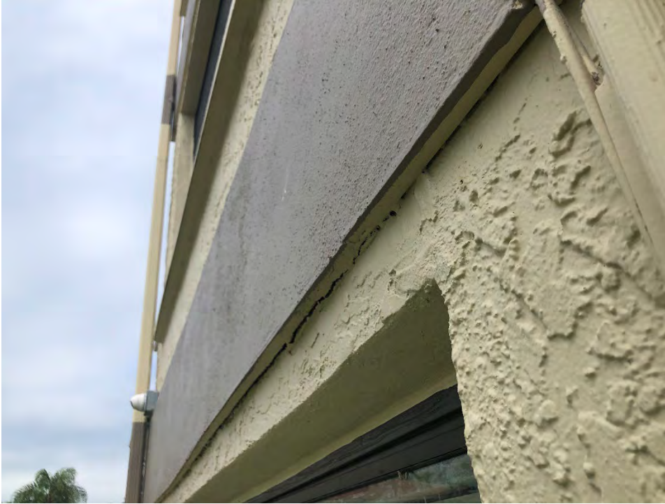
Figure E- 73 – Typical Separation at Stucco Banding
