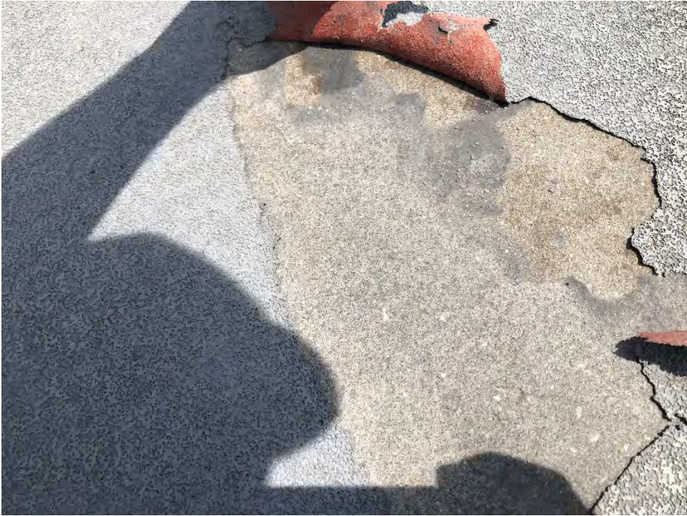
Figure D- 5 – Peeling Waterproofing Membrane
