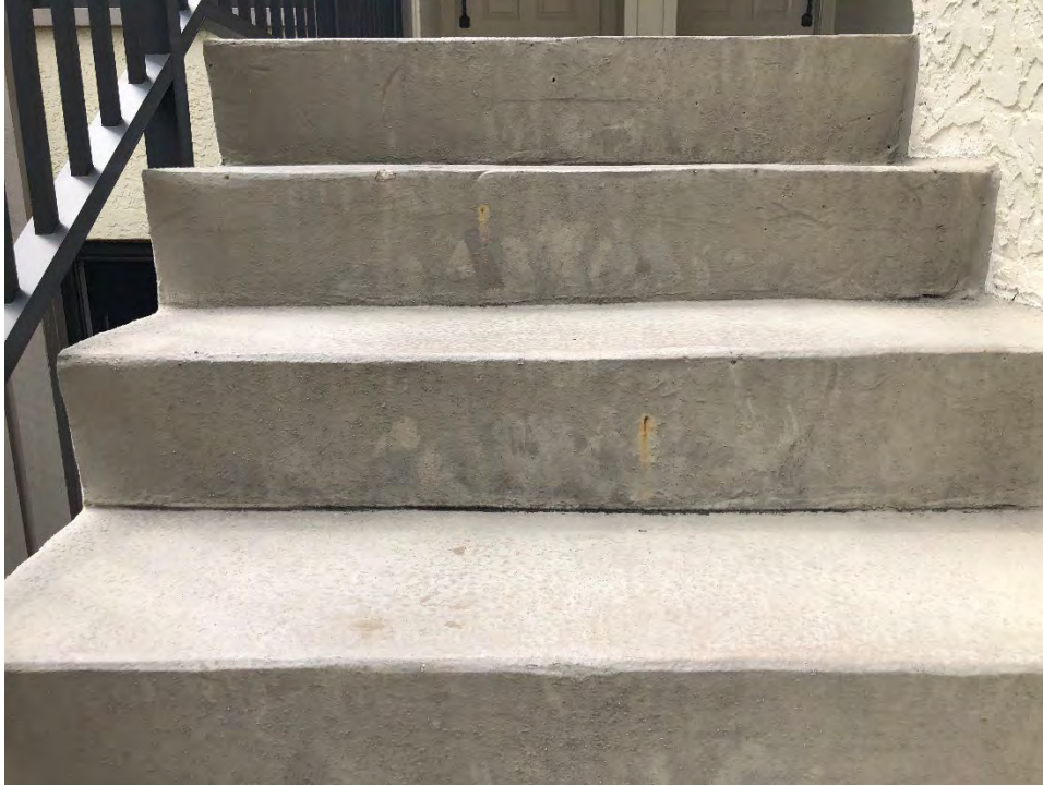
Figure B- 19 – Floor Staining
