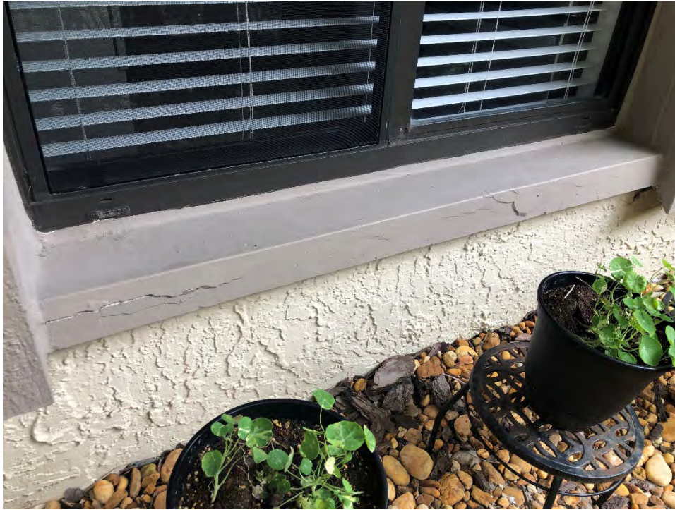
Figure E- 47 – Windowsill Spall (Unit 110)
