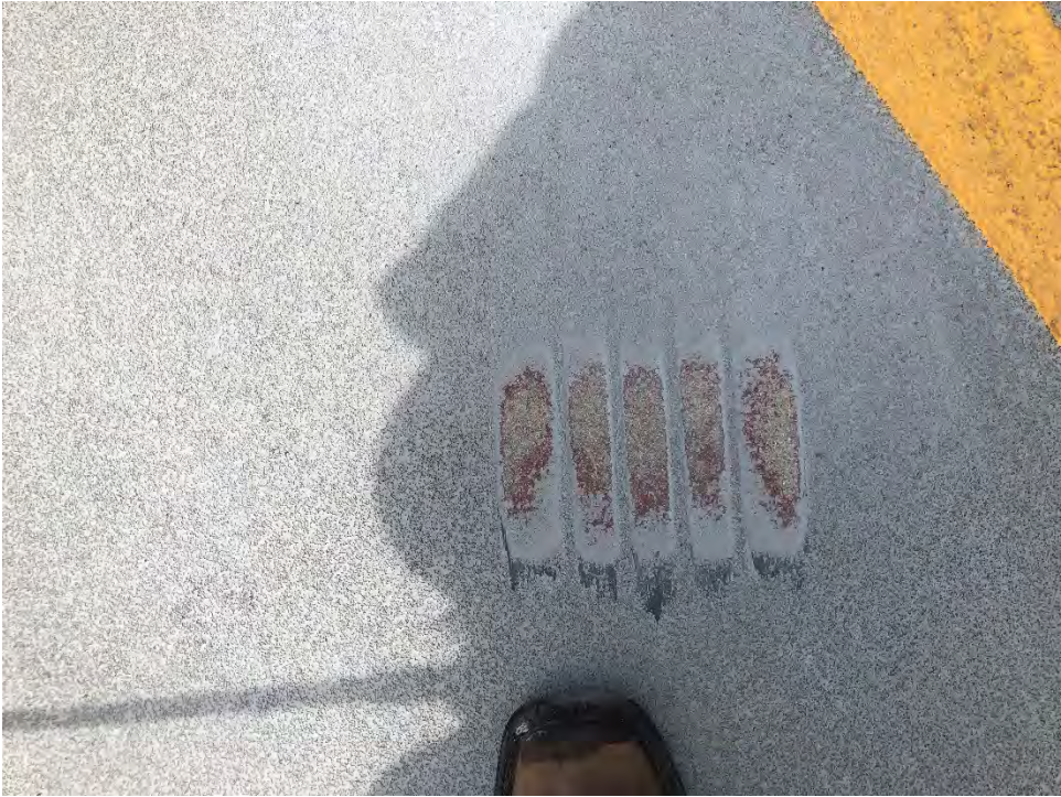
Figure D- 6 – Scraped Waterproofing Membrane
