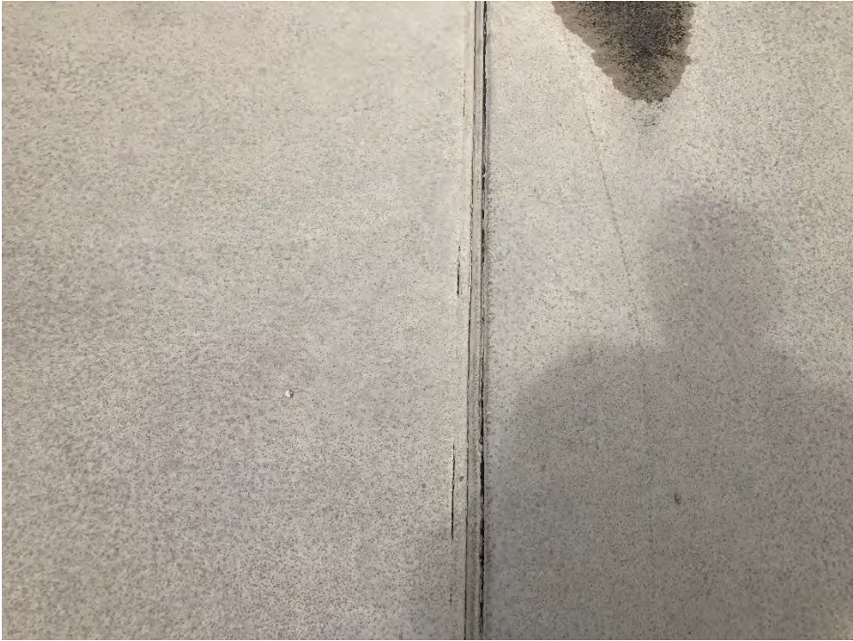
Figure B- 16 – Deteriorated/Failed Expansion Joint
