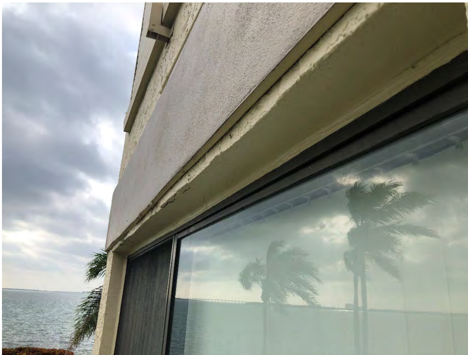
Figure A- 14 – Unit 204 Concrete Lintel Spall
