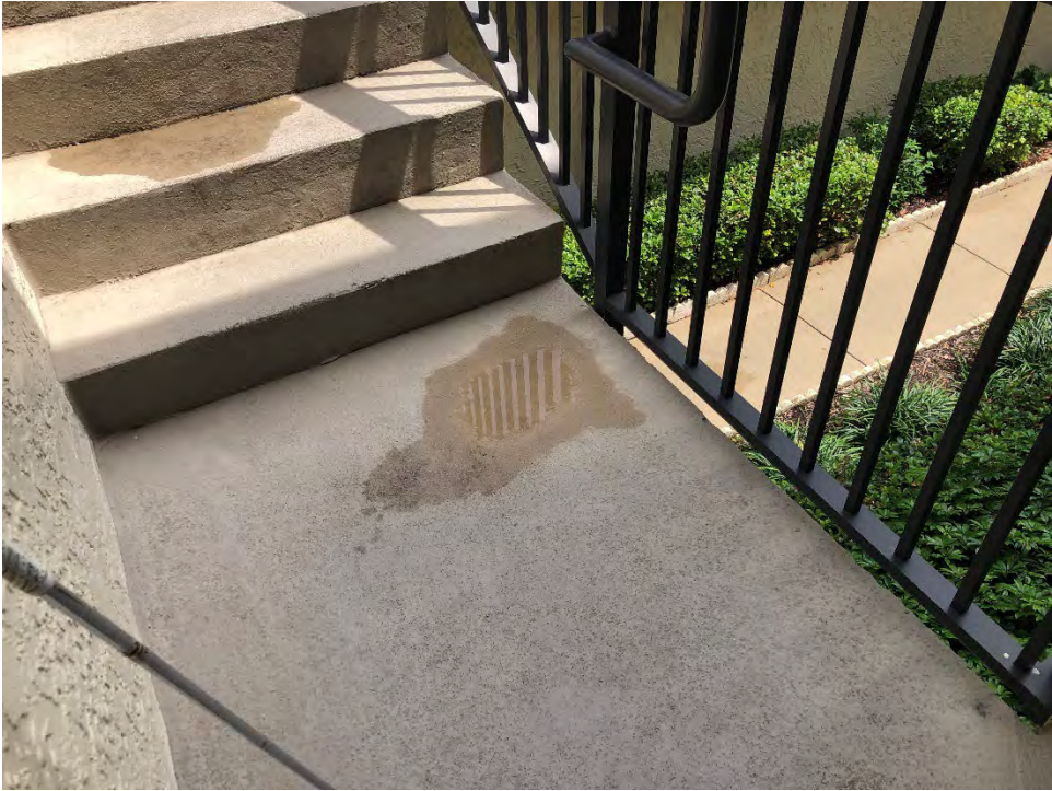
Figure B- 14 – Ponding Water
