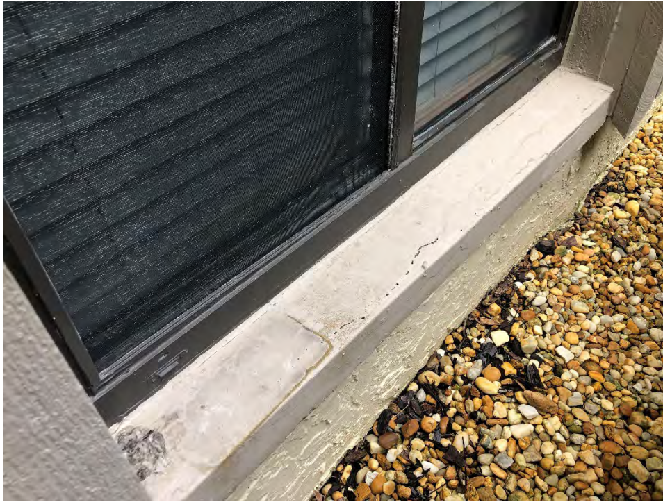
Figure E- 51 – Windowsill Spall (Unit 116)
