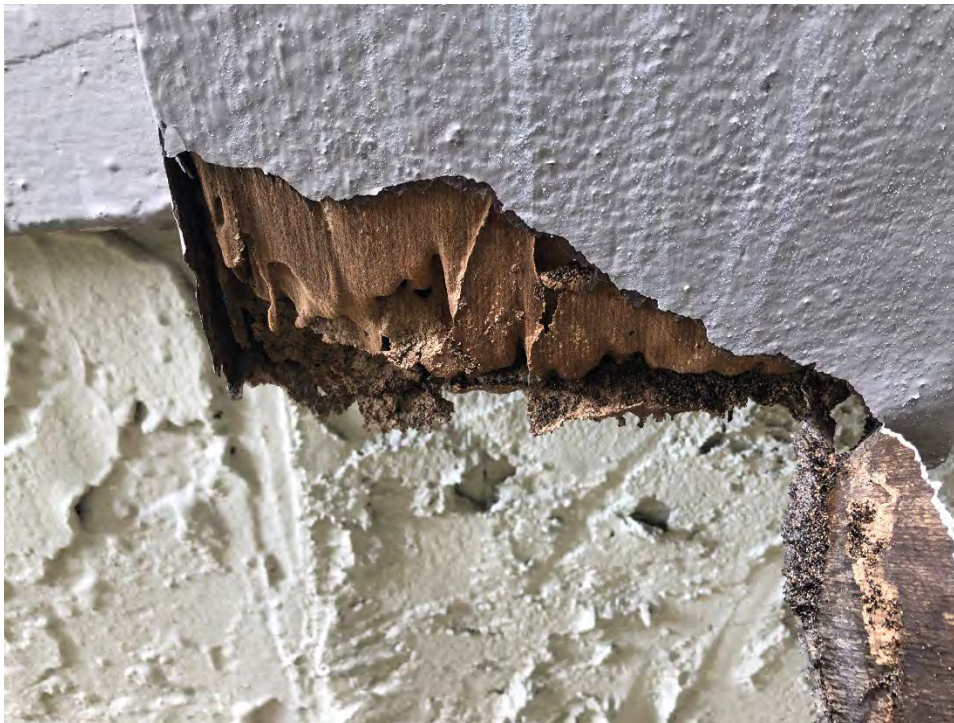
Figure E- 68 – Typical Wood Trim Rot
