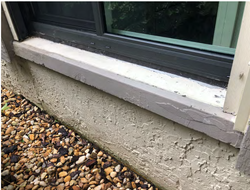
Figure E- 42 – Windowsill Spall (Unit 105)
