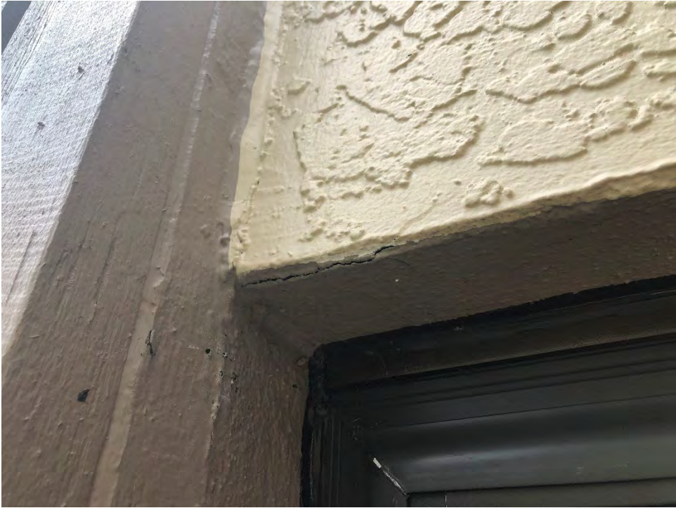
Figure E- 62 – Concrete Lintel Spall (Unit 113)
