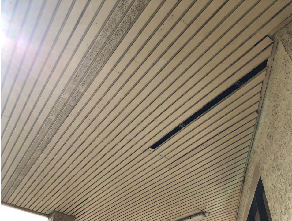
Figure E- 7 – Missing Soffit
