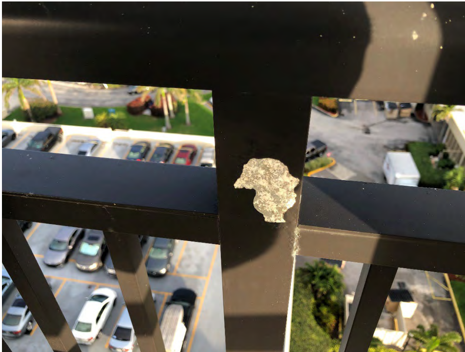
Figure A- 4 – Typical Tower Guardrail Peeling Paint/Oxidization
