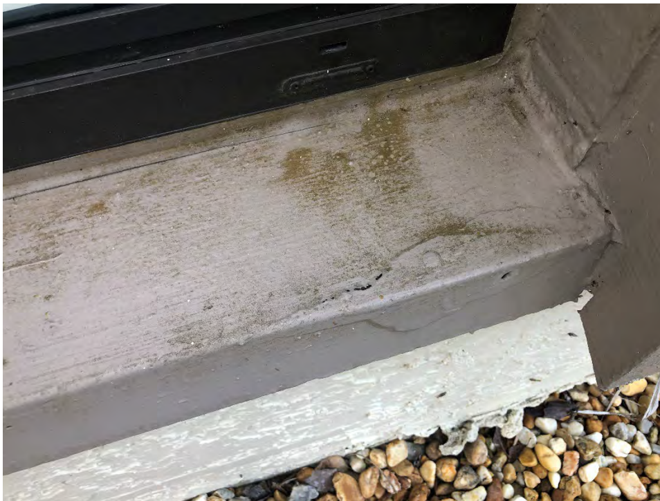
Figure E- 52 – Windowsill Spall (Unit 120)
