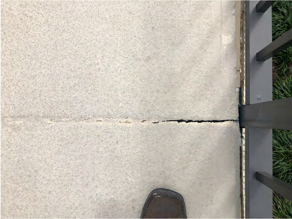
Figure B- 15 – Deteriorated/Failed Expansion Joint
