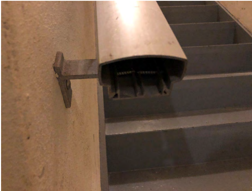
Figure C- 4 – Missing Handrail End Cap
