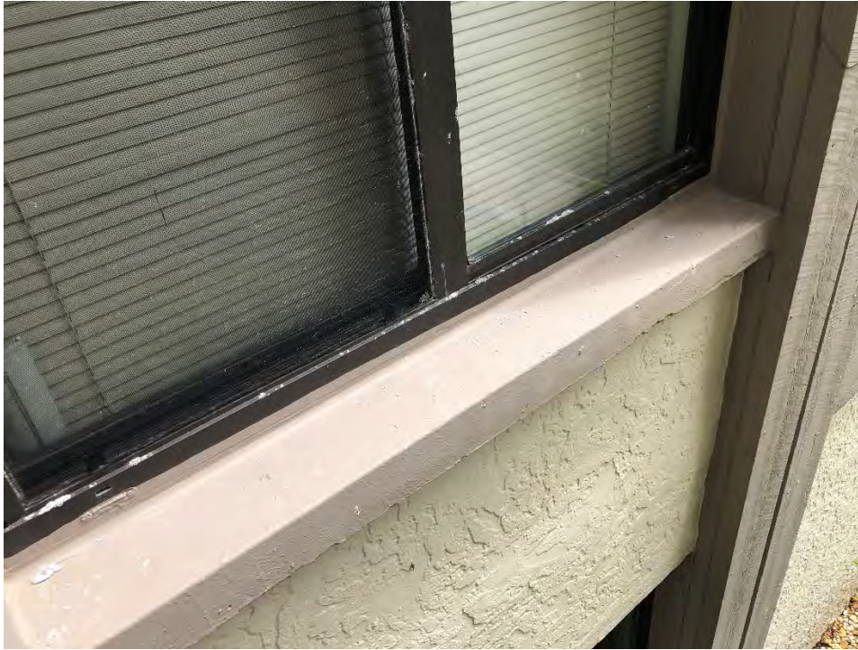
Figure E- 39 – Windowsill Spall (Unit 204)
