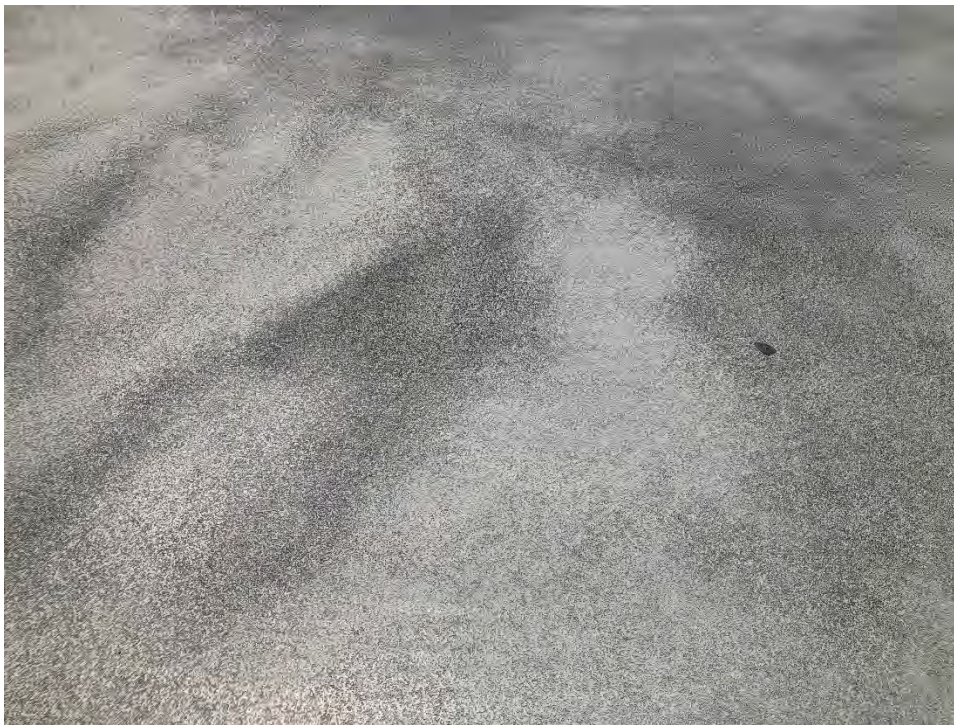
Figure D- 4 – Worn/Deteriorated Waterproofing Membrane
