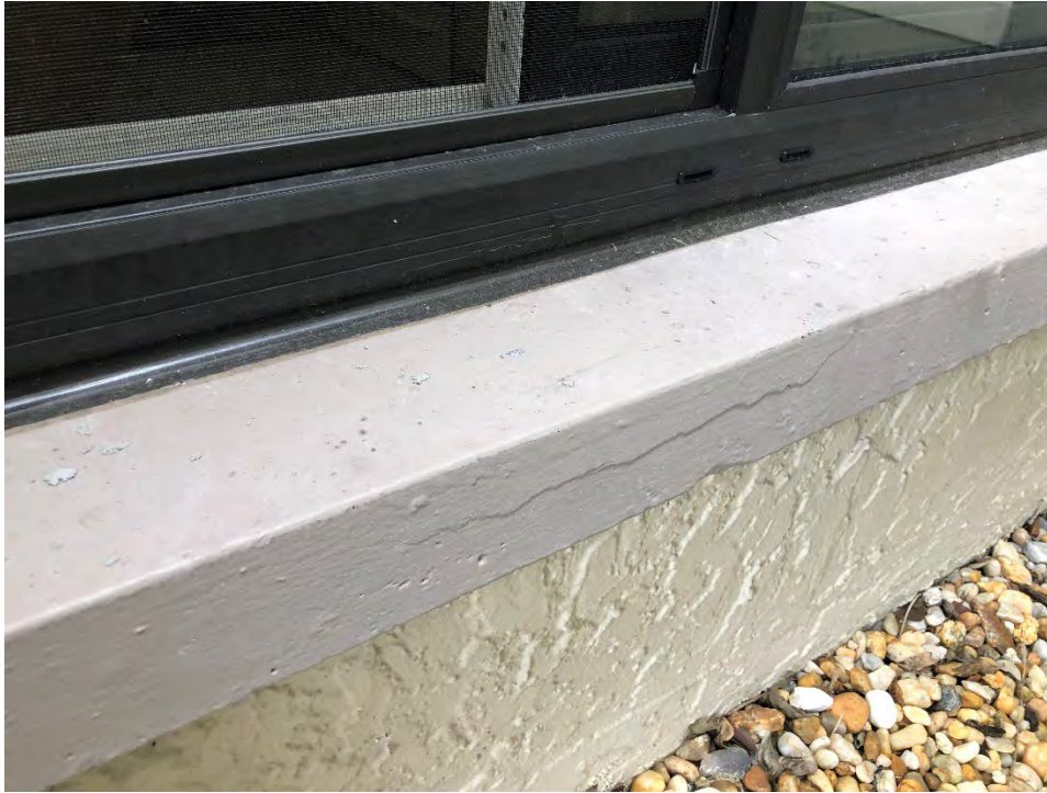
Figure E- 33 – Windowsill Spall (Unit 102)
