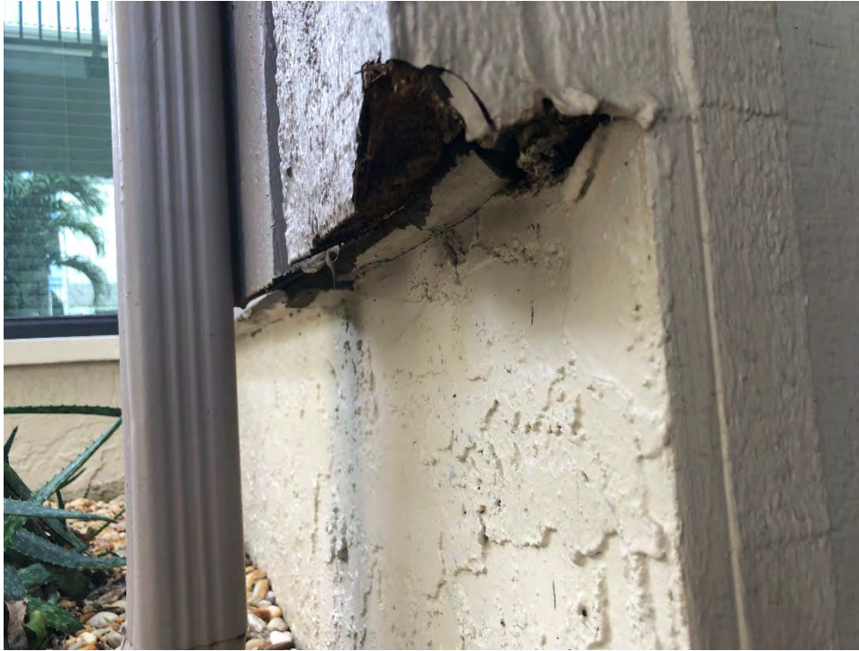
Figure E- 69 – Typical Wood Trim Rot
