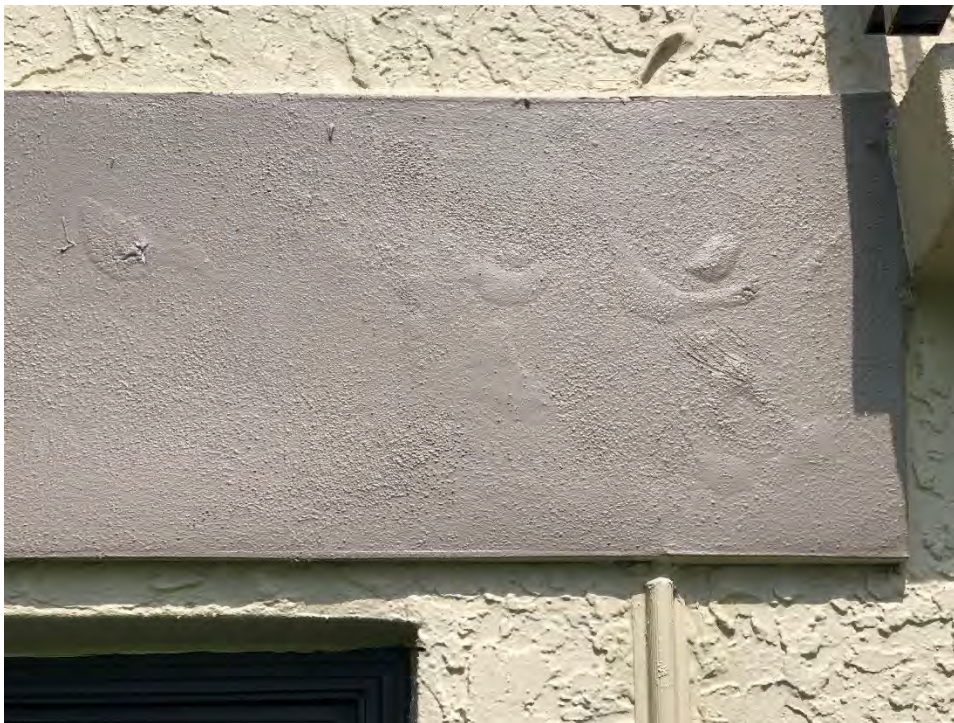
Figure E- 64 – Blistering Exterior Paint Coatings
