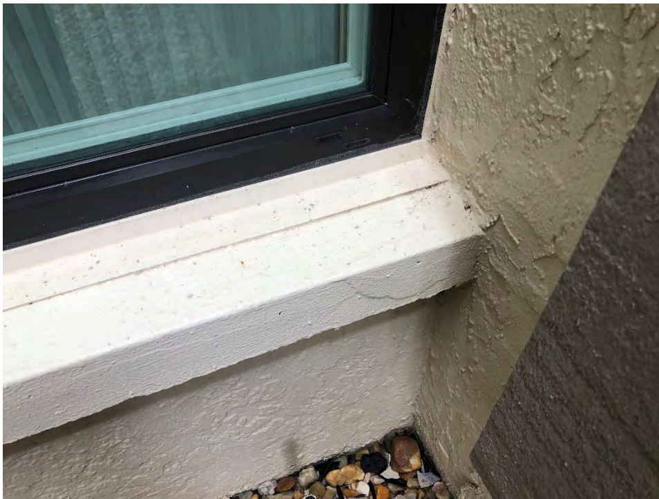
Figure E- 34 – Windowsill Spall (Unit 103)
