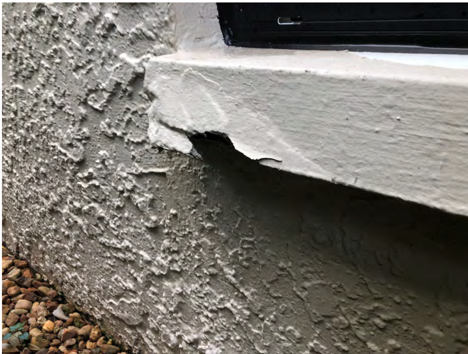
Figure E- 46 – Windowsill Spall (Unit 109)
