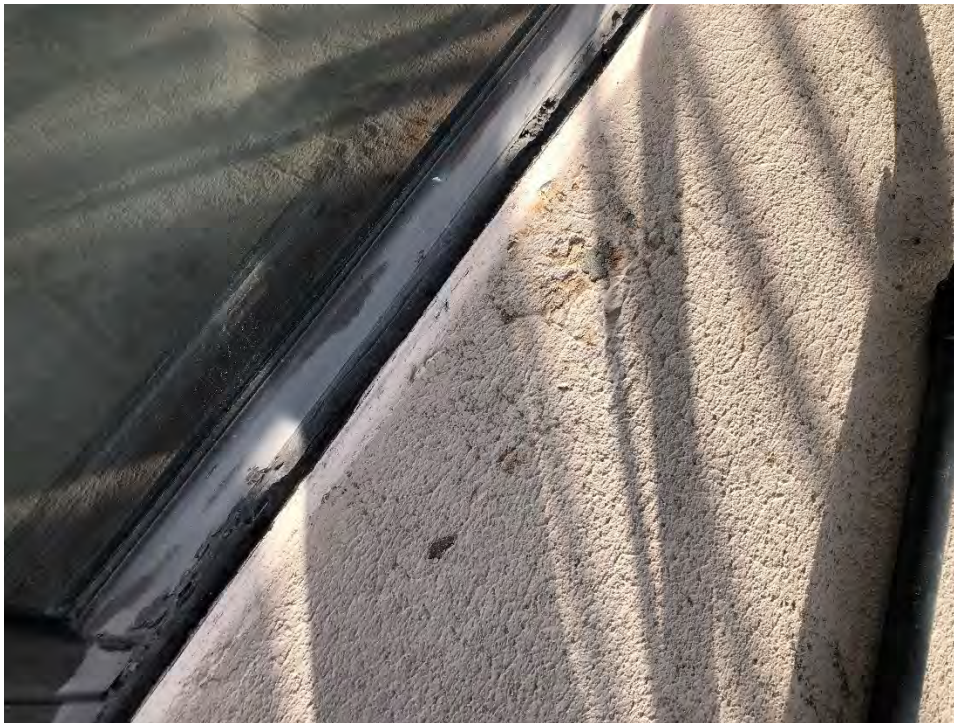
Figure A- 8 – Unit 906 Area of Unsound Concrete/Concrete Spall
