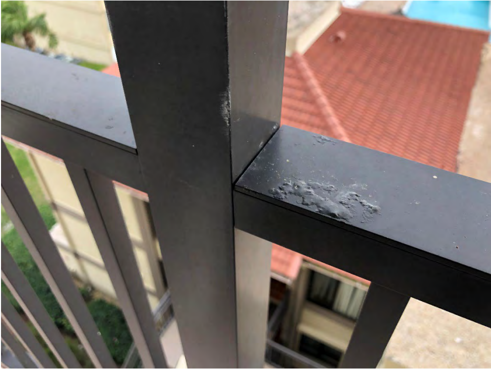
Figure A- 6 – Typical Tower Guardrail Peeling Paint/Oxidization
