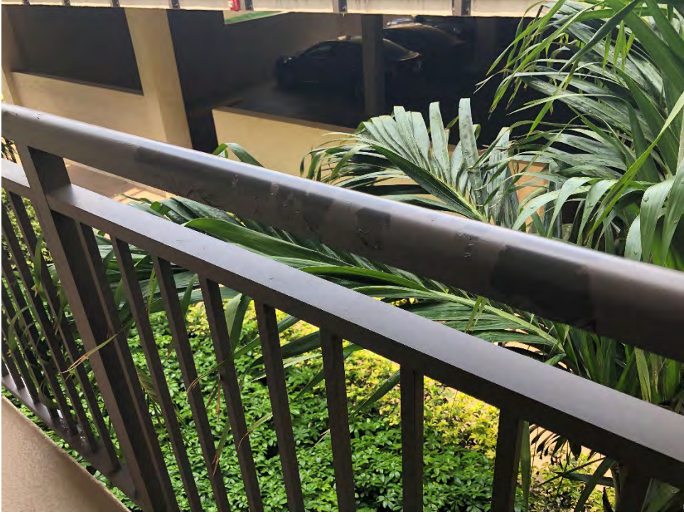
Figure B- 10 – Typical Guardrail Peeling Paint
