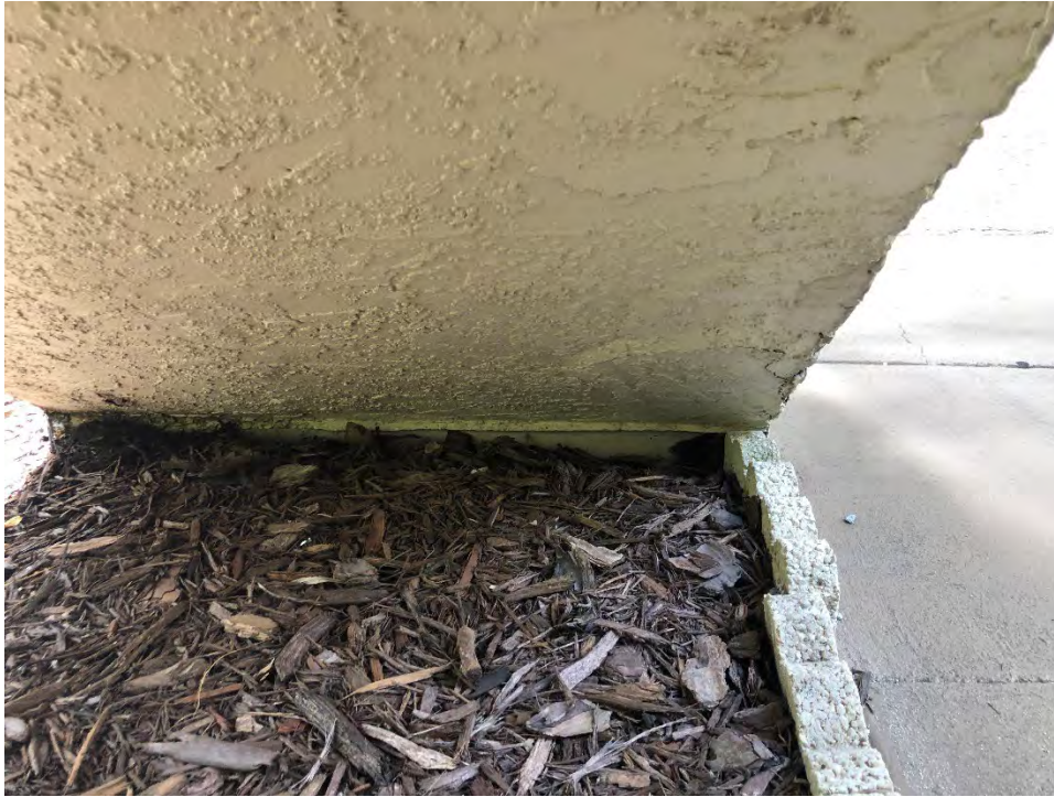
Figure B- 23 – Concrete Spall
