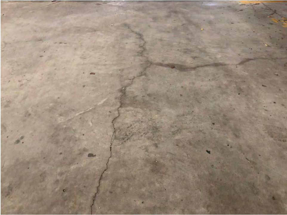
Figure D- 26 – Concrete Slab Cracks
