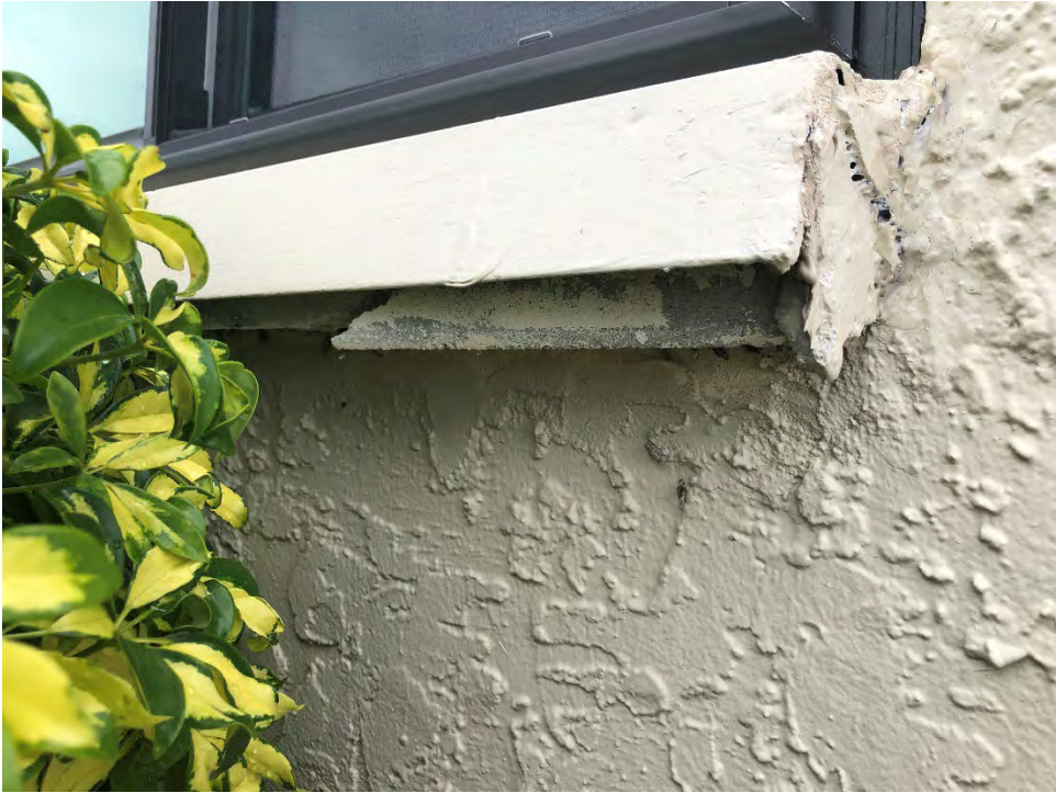
Figure E- 49 – Windowsill Spall (Unit 113)
