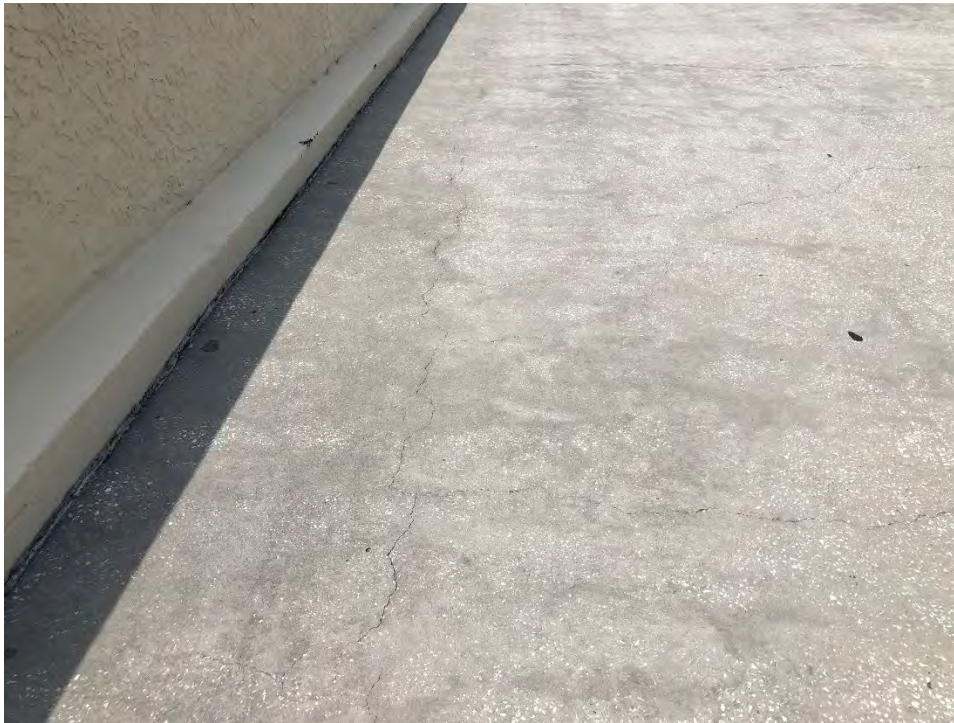
Figure D- 18 – Concrete Slab Cracks
