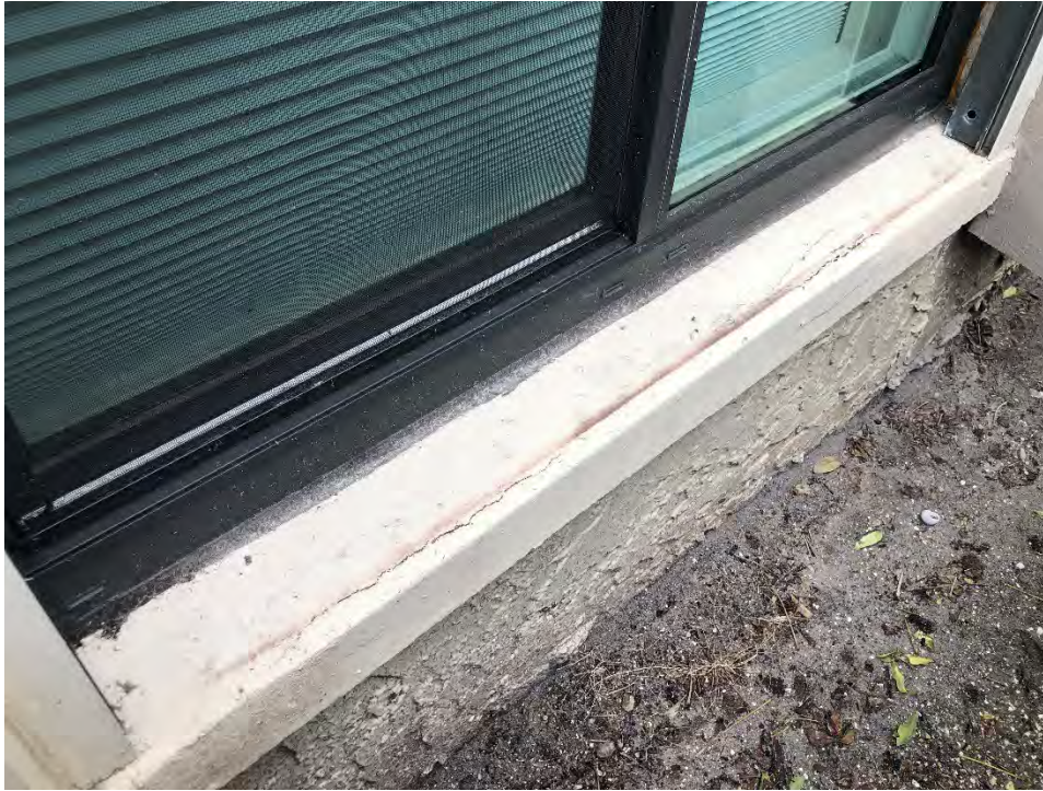
Figure E- 41 – Windowsill Spall (Unit 105)
