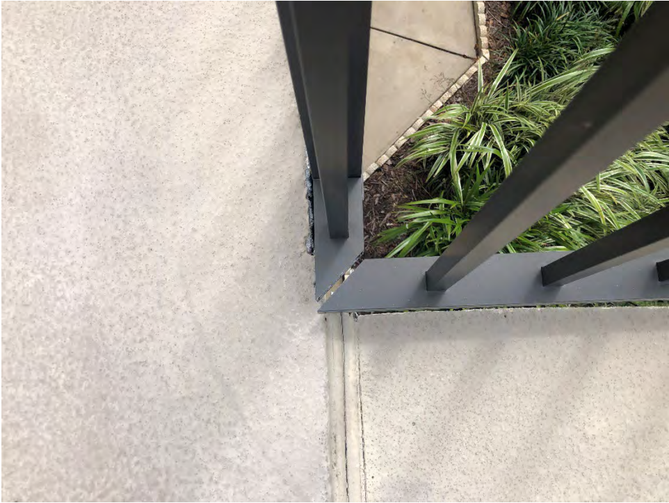
Figure B- 18 – Loose Bottom Rail Connection
