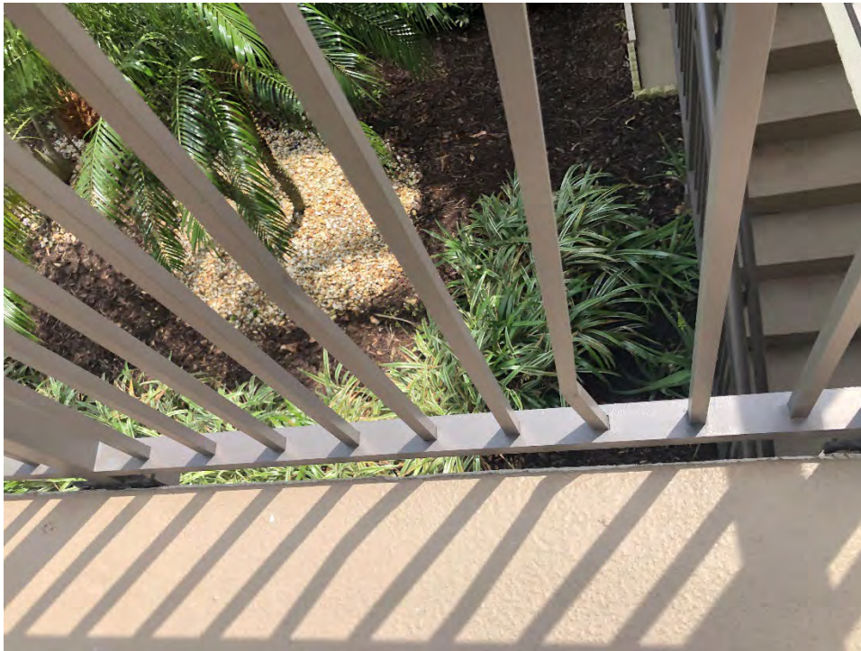
Figure B- 20 – Bent Guardrail Picket
