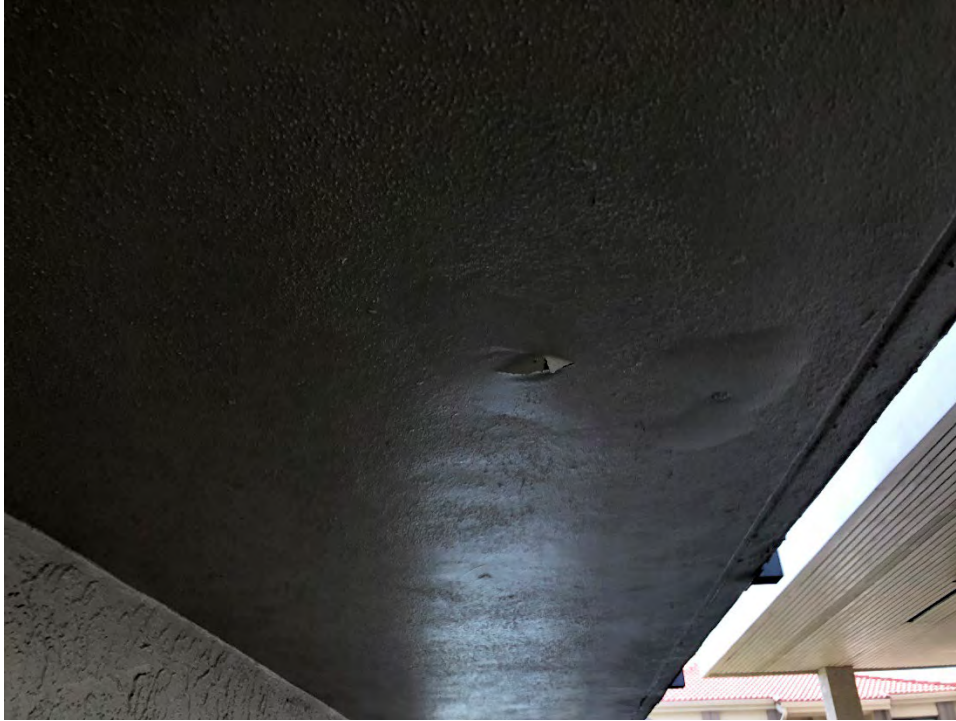
Figure B- 27 – Blistering Paint Coatings
