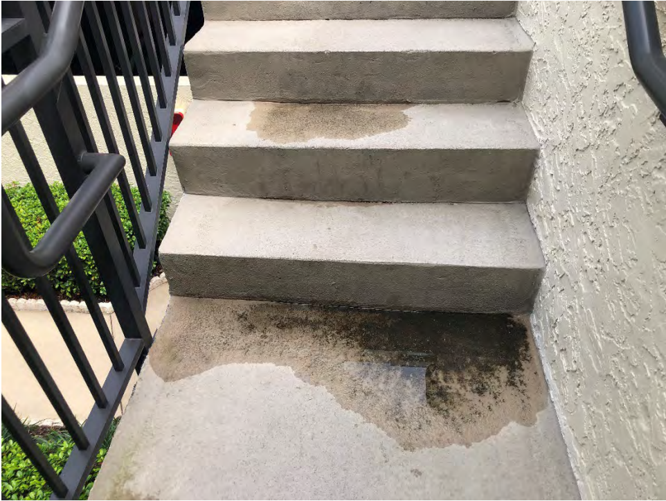
Figure B- 12 – Ponding Water
