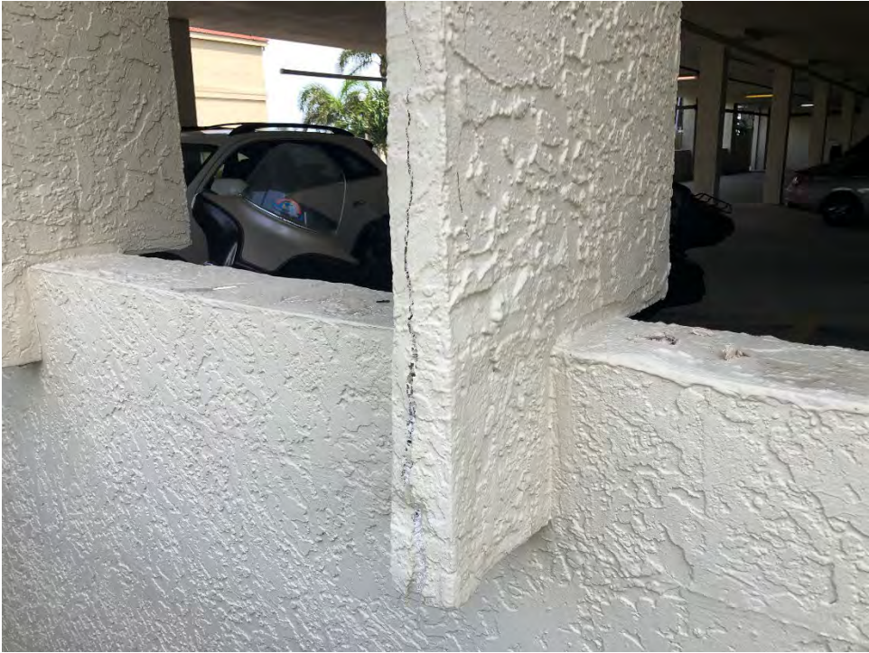
Figure D- 20 – Concrete Spall
