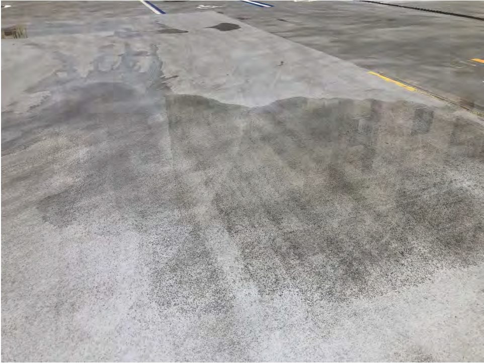
Figure D- 7 – Ponding Water
