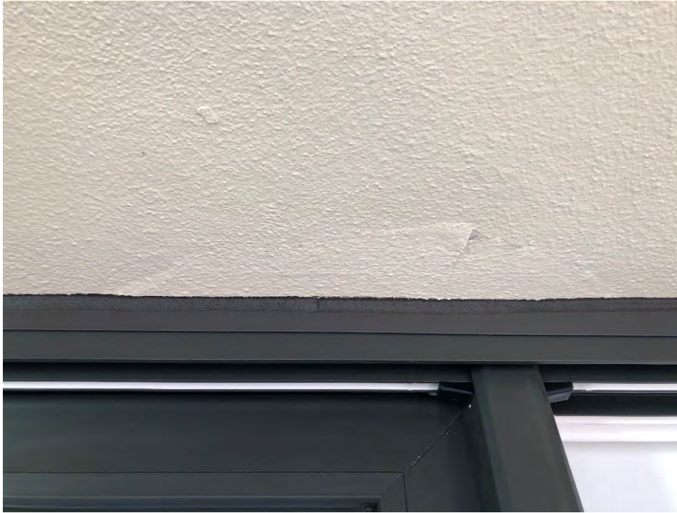
Figure A- 9 – Unit 1106 Delaminated Exterior Stucco Ceiling Finishes
