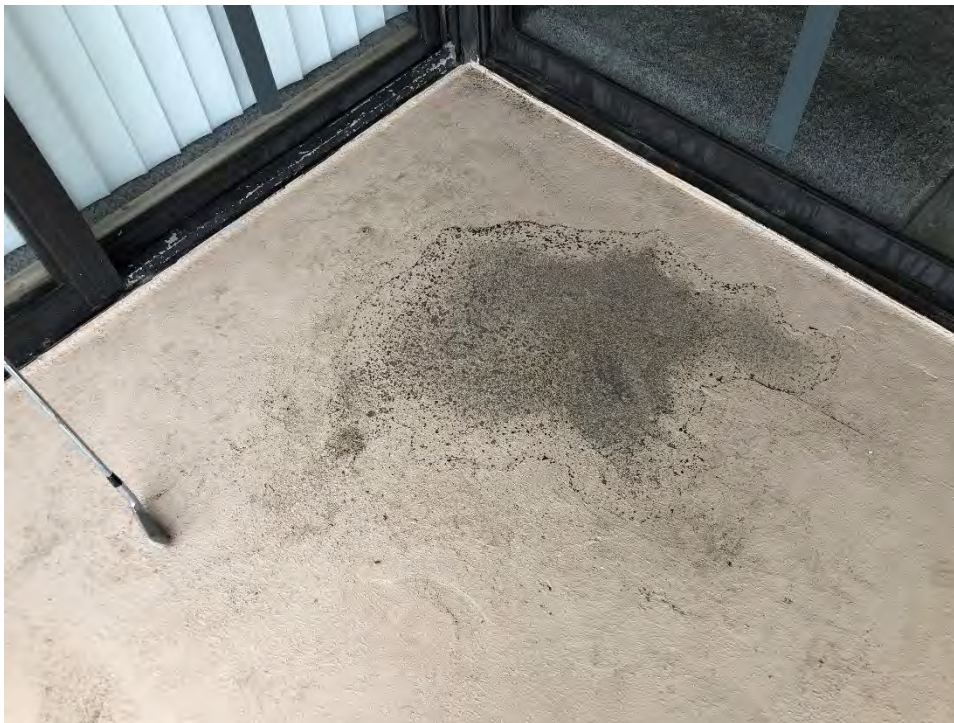
Figure A- 10 – Unit 704 Ponding Water Stains
