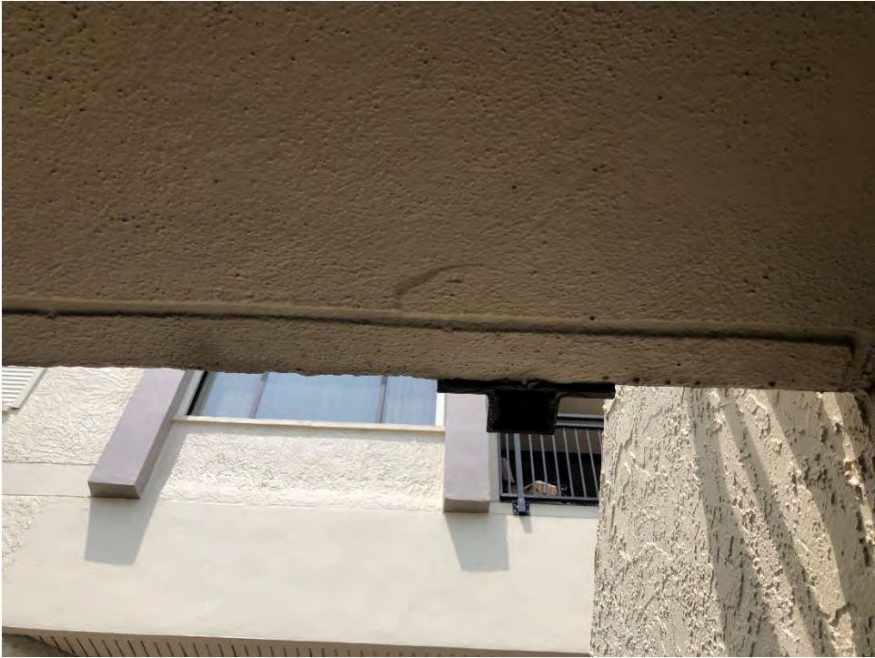
Figure B- 21 – Concrete Spall
