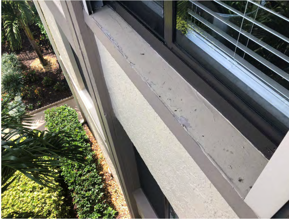
Figure E- 65 – Peeling Exterior Paint Coatings
