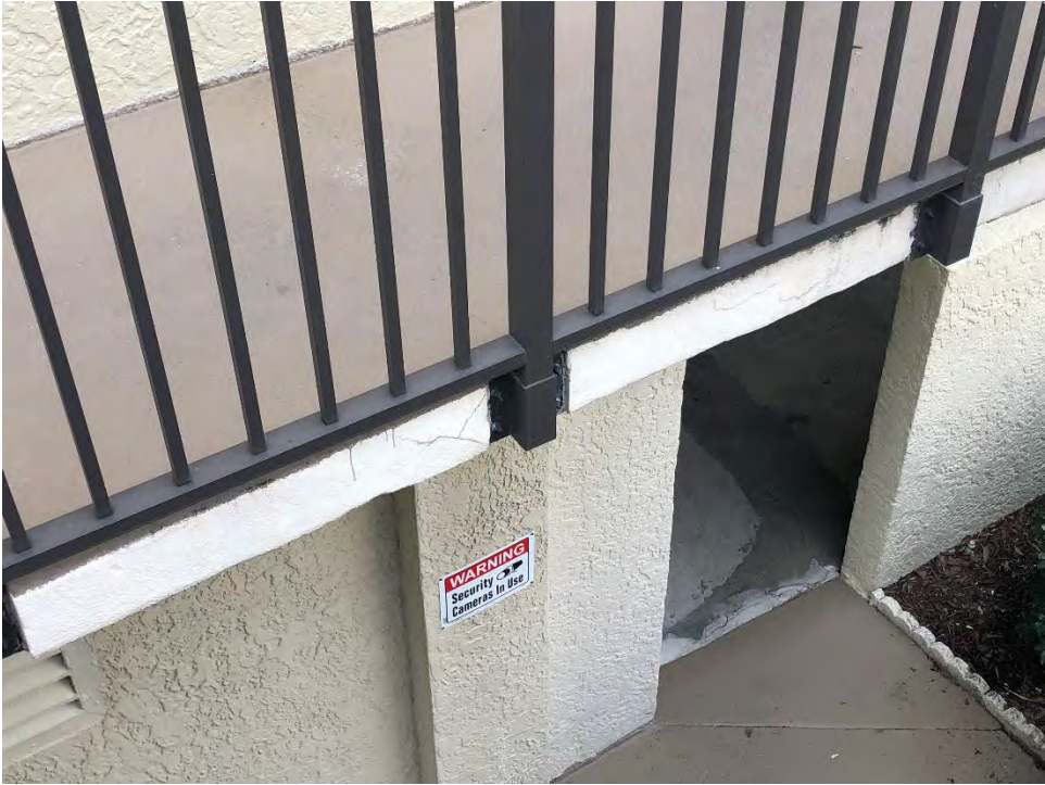
Figure B- 22 – Concrete Spall
