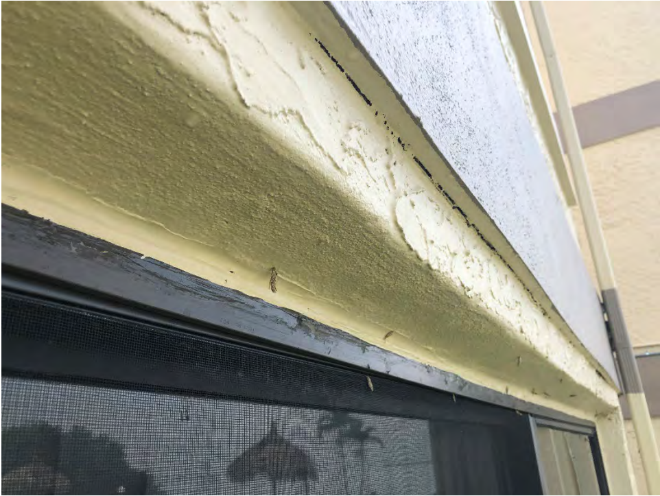
Figure E- 72 – Typical Separation at Stucco Banding
