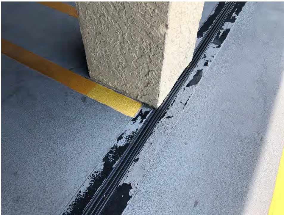
Figure D- 16 – Deteriorated/Peeling Waterproofing Membrane
