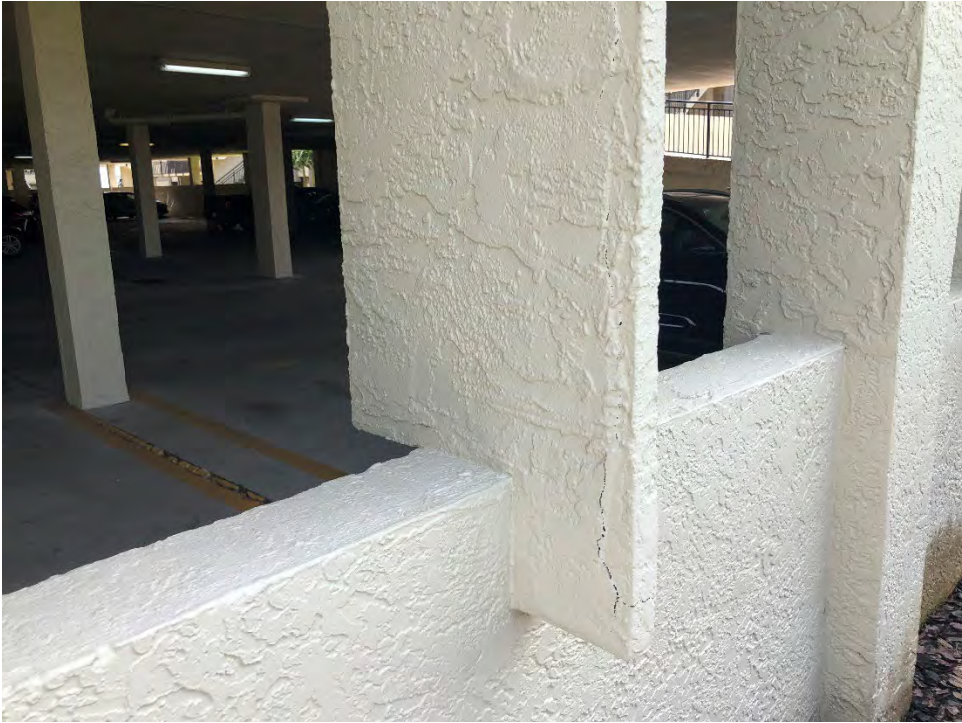
Figure D- 22 – Concrete Spall
