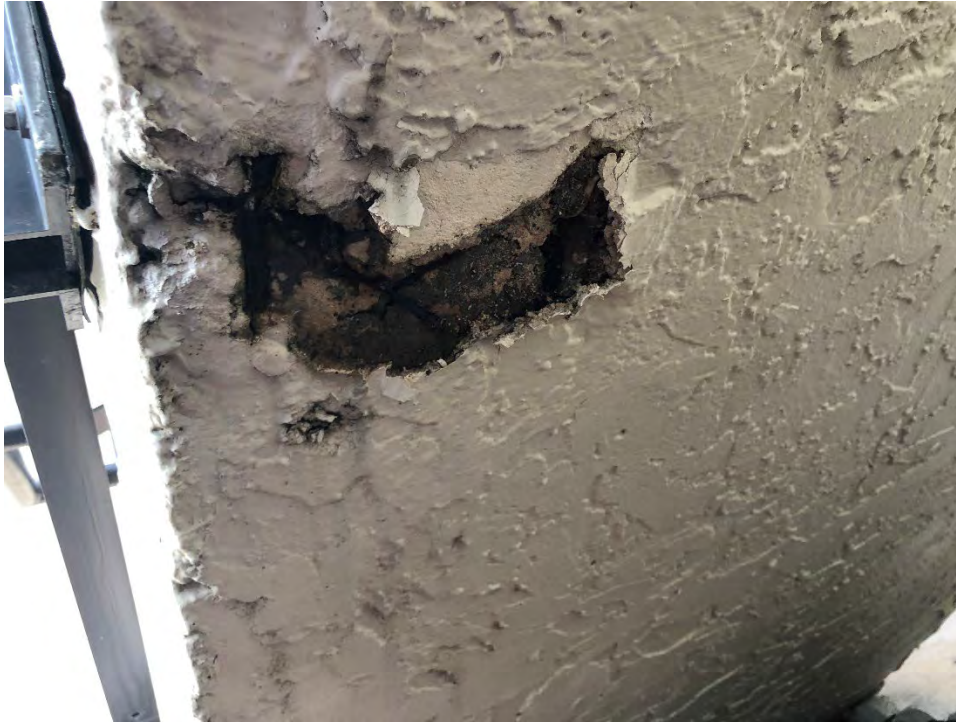
Figure B- 25 – Concrete Spall
