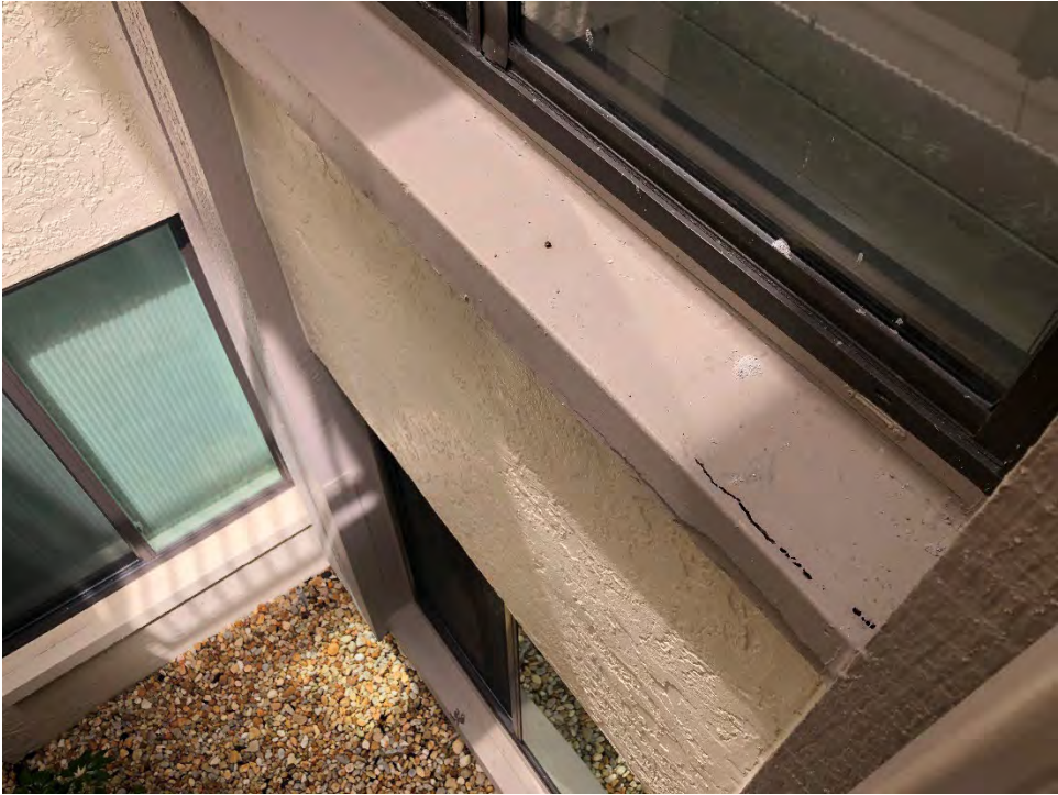
Figure E- 38 – Windowsill Spall (Unit 203)
