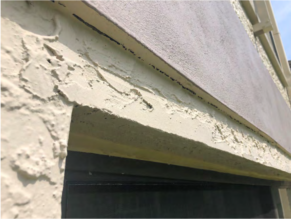
Figure E- 71 – Typical Separation at Stucco Banding
