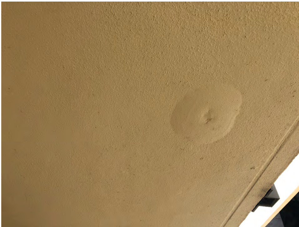
Figure B- 26 – Blistering Paint Coatings
