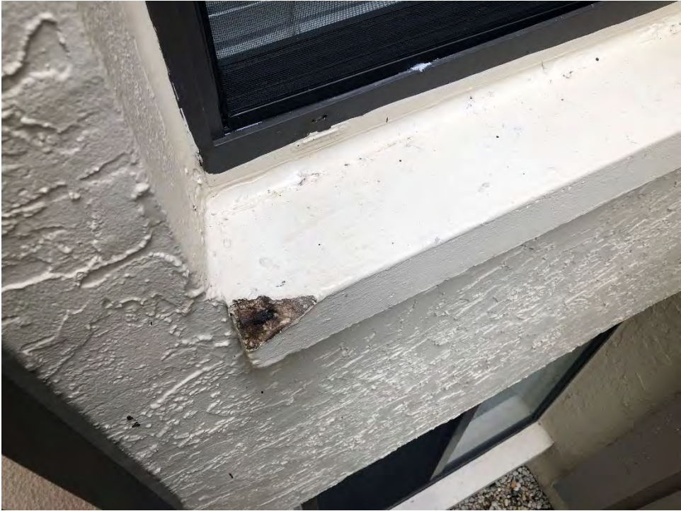
Figure E- 44 – Windowsill Spall (Unit 207)
