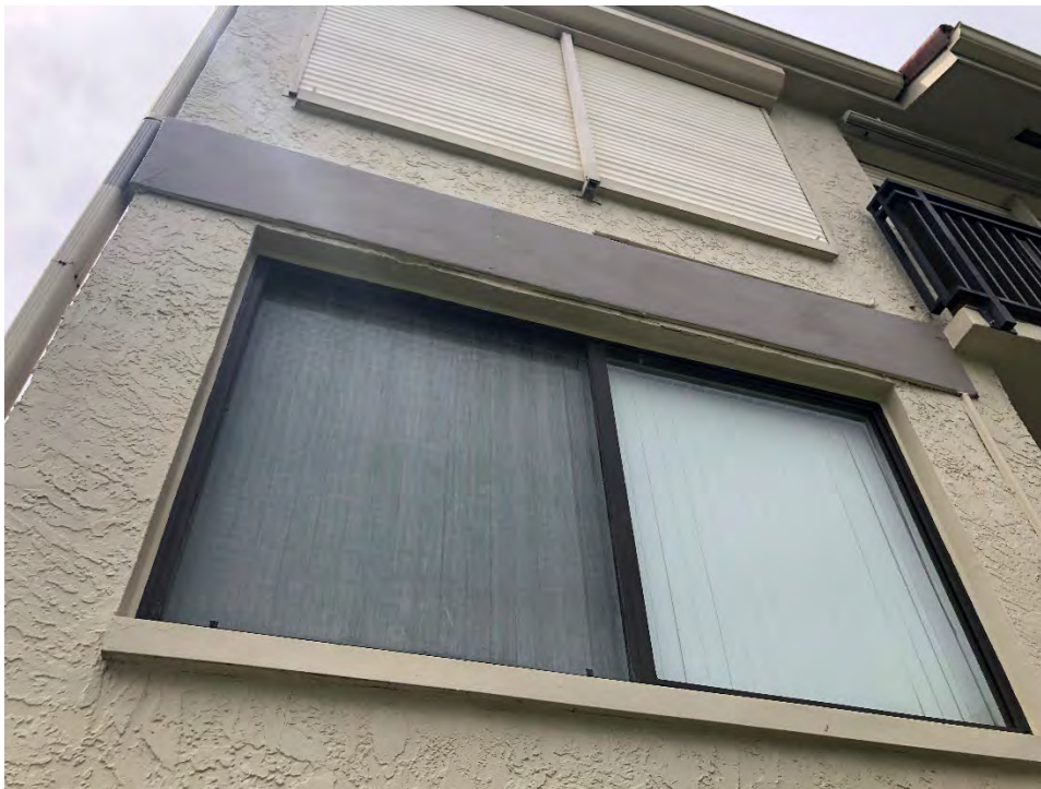
Figure E- 60 – Concrete Lintel Spall (Unit 204)
