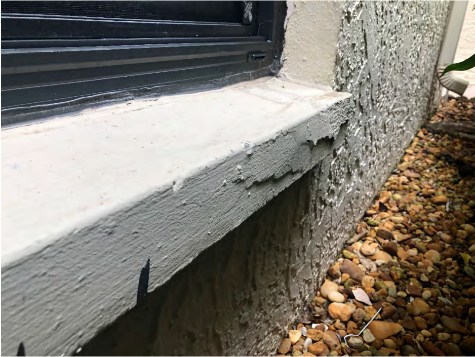
Figure E- 43 – Windowsill Spall (Unit 108)
