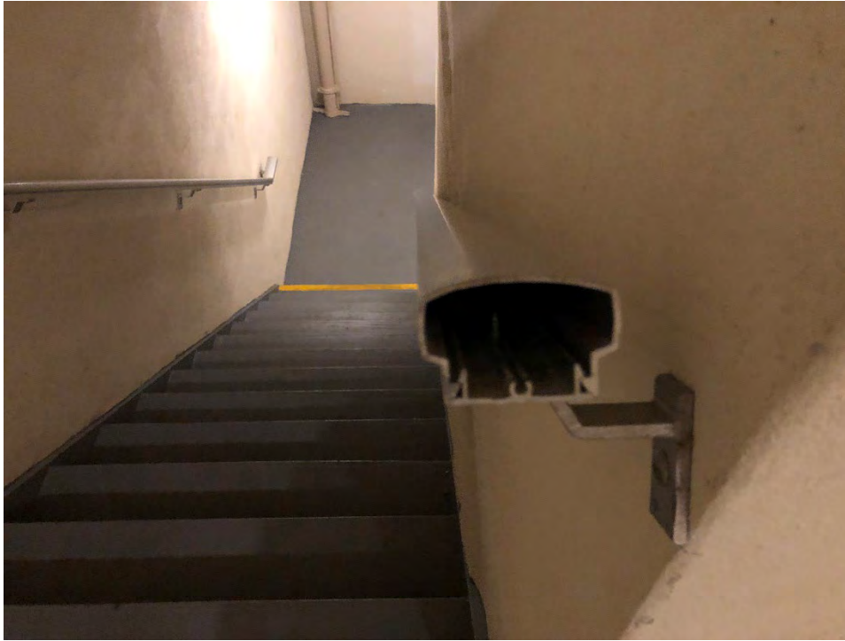
Figure C- 5 – Missing Handrail End Cap
