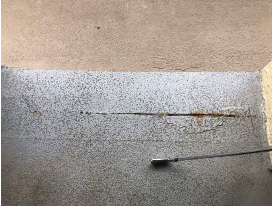
Figure D- 17 – Concrete Spall
