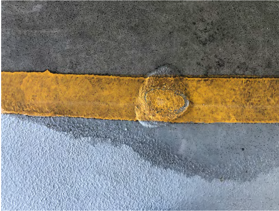
Figure D- 15 – Concrete Spall
