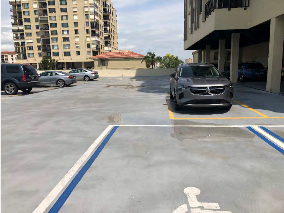
Figure D- 8 – Ponding Water
