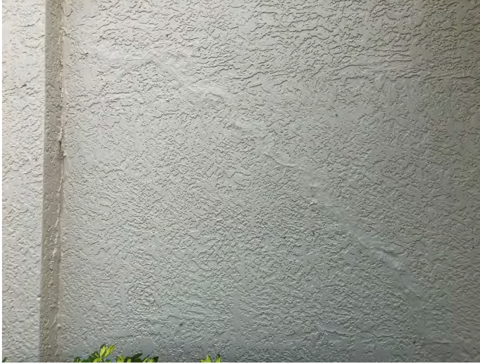
Figure D- 23 – Exterior Wall Crack
