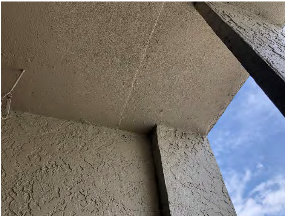
Figure D- 24 – Concrete Spall
