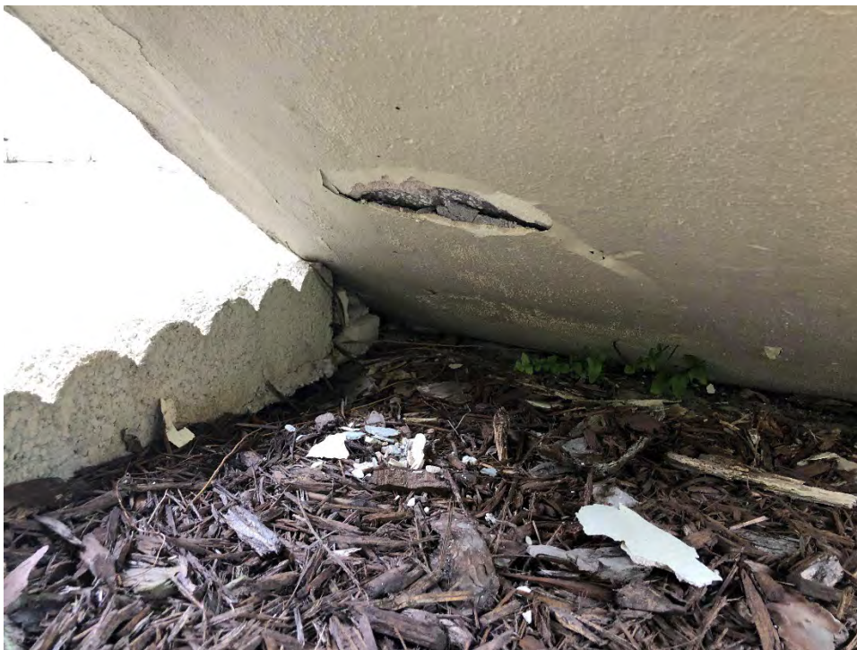
Figure B- 24 – Concrete Spall
