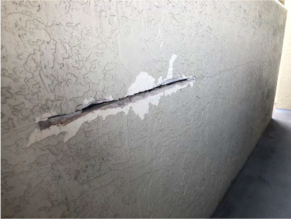
Figure D- 14 – Exposed Rusting Metal and Delaminated Stucco
