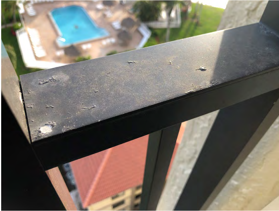
Figure A- 7 – Typical Tower Guardrail Peeling Paint/Oxidization
