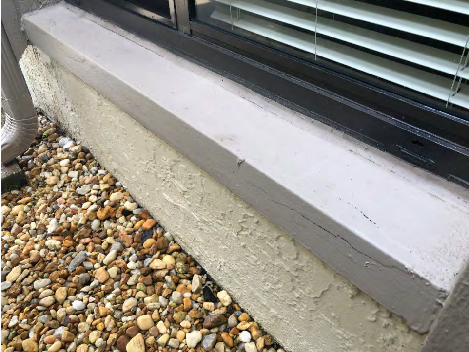
Figure E- 50 – Windowsill Spall (Unit 114)
