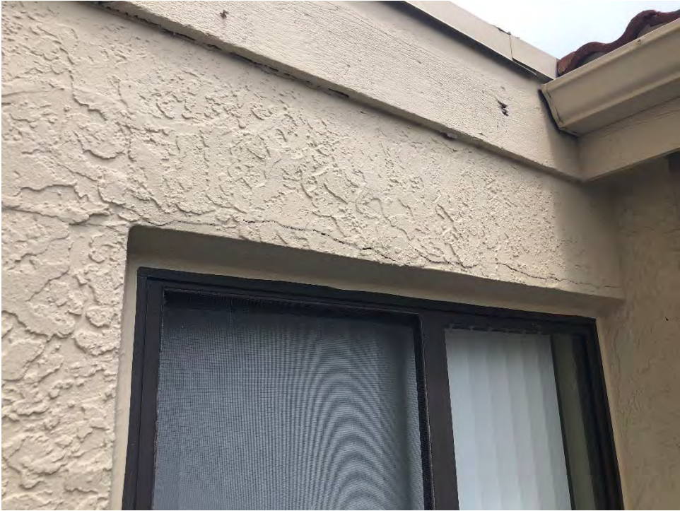
Figure E- 61 – Concrete Lintel Spall (Unit 303)
