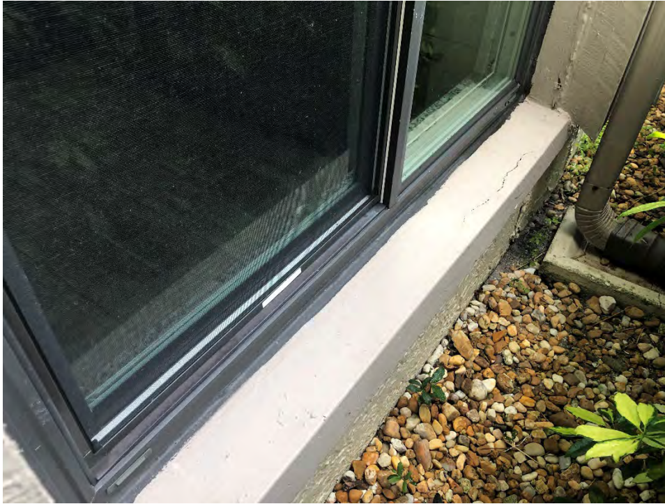
Figure E- 53 – Windowsill Spall (Unit 223)
