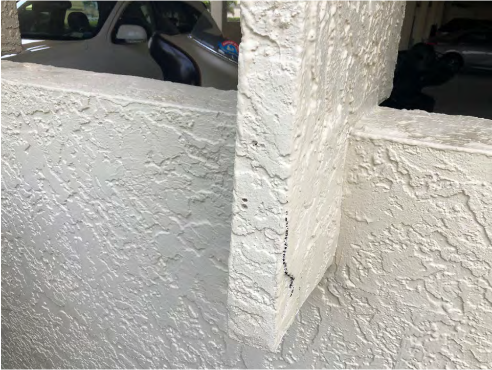
Figure D- 21 – Concrete Spall
