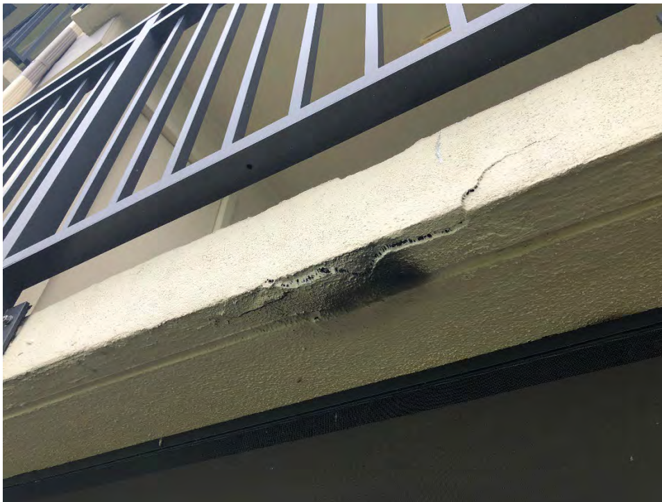
Figure E- 70 – Concrete Spall (Unit 209)
