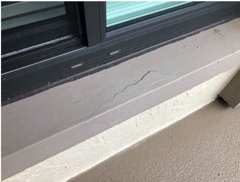
Figure E- 48 – Windowsill Spall (Unit 210)
