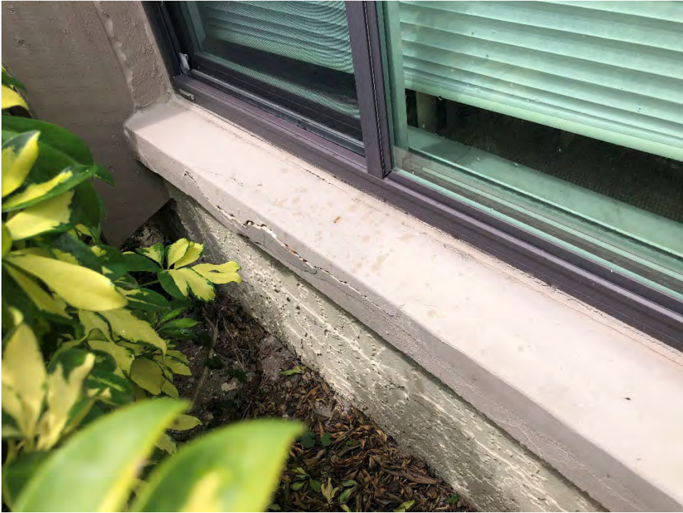
Figure E- 36 – Windowsill Spall (Unit 104)
