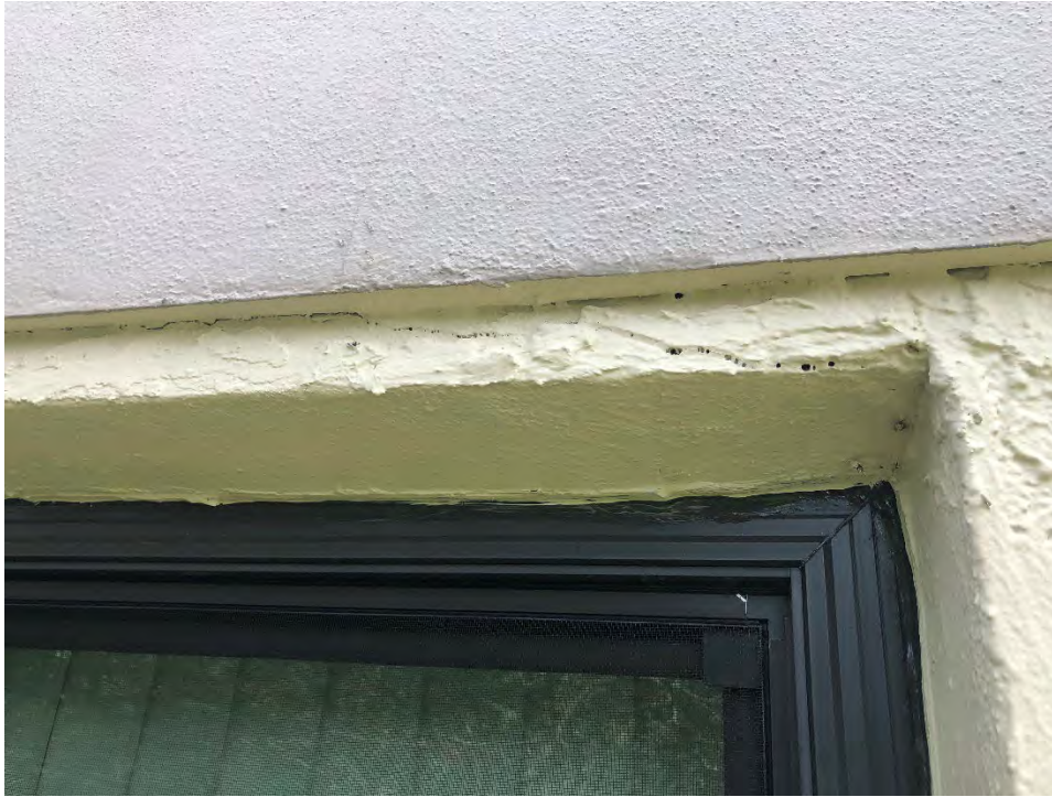
Figure E- 63 – Concrete Lintel Spall (Unit 120)
