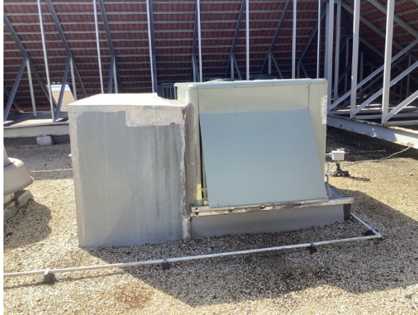
Roof top unit
