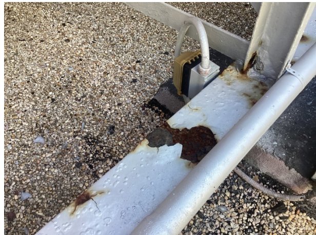
Steel structure – corrosion evident
