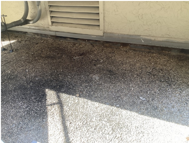
Built-up roof – granular loss evident
