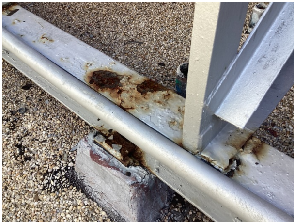
Steel structure – corrosion evident
