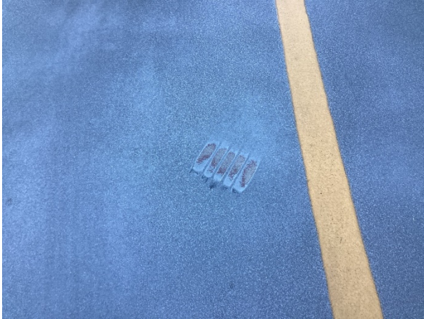
Traffic coating – deterioration evident
