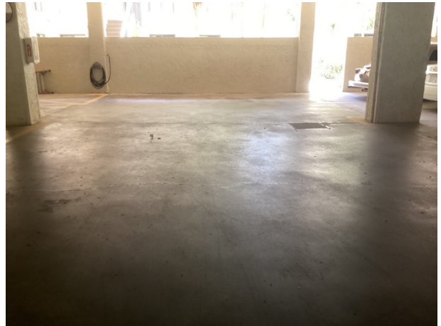
On grade concrete – cracks evident
