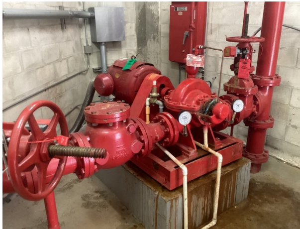
Fire pump - overview
