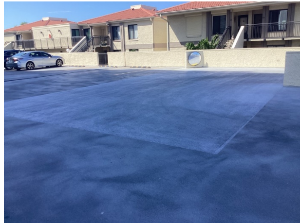
Traffic coating – deterioration evident
