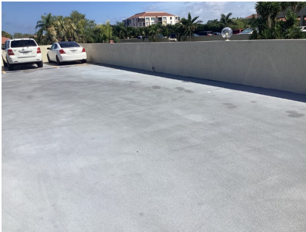
Traffic coating – deterioration evident
