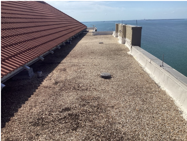
Built-up roof – granular loss evident
