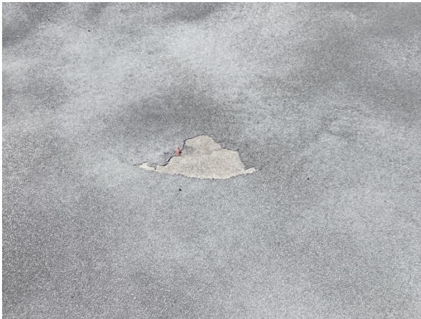
Traffic coating – deterioration evident
