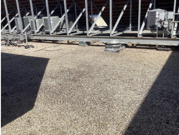
Built-up roof – granular loss evident
