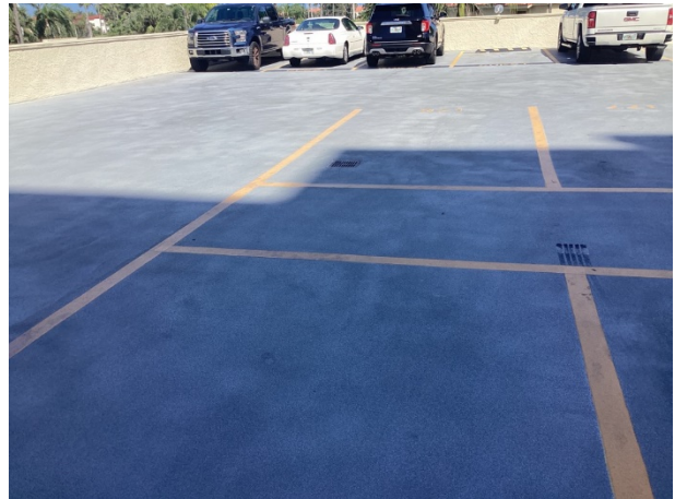
Traffic coating – deterioration evident
