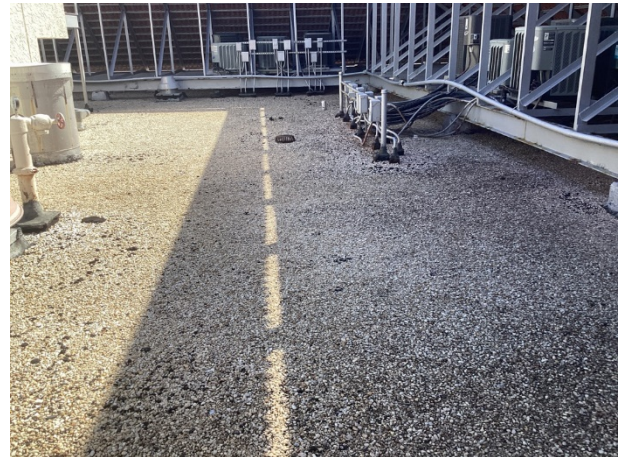
Built-up roof – granular loss evident
