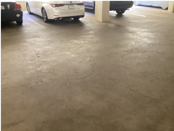
On grade concrete – cracks evident
