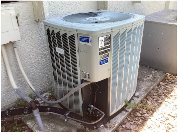
Split systems – overview
