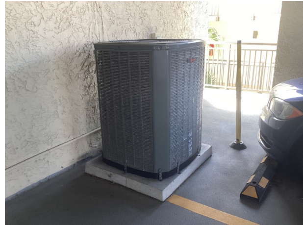
Split systems - overview
