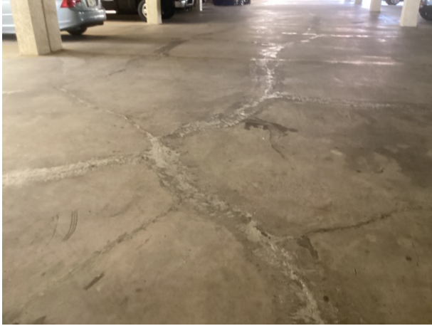
On grade concrete – cracks evident
