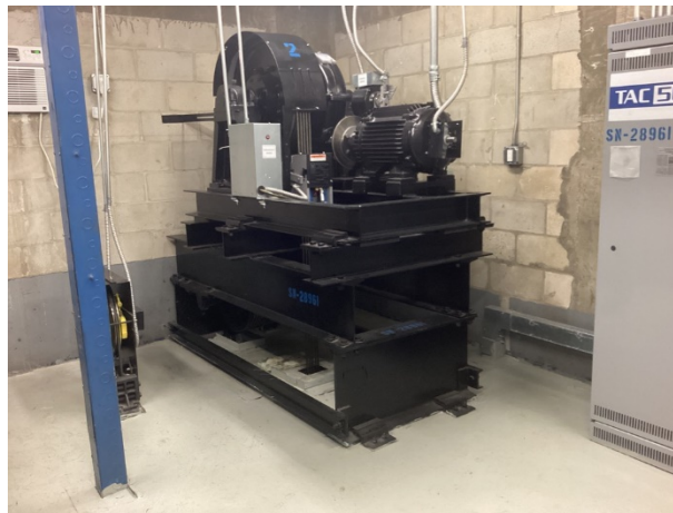
Elevator equipment - hoists
