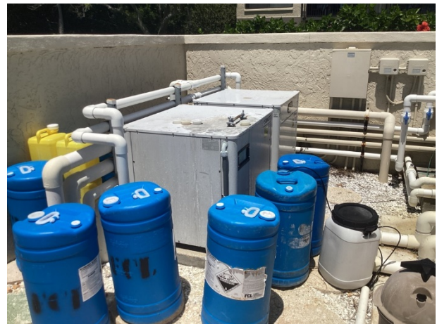
Pool mechanical equipment – geothermal heaters
