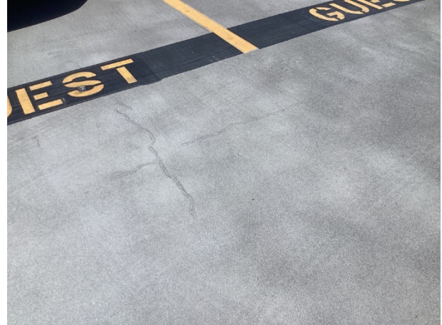
Elevated concrete – cracks evident
