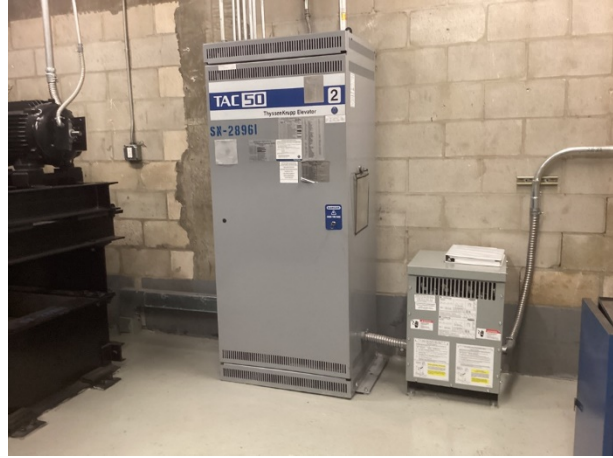
Elevator equipment – control panel
