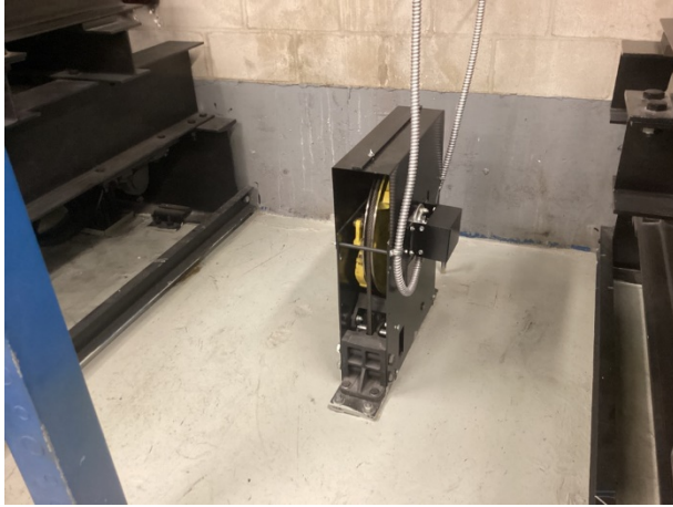
Elevator equipment - hoists
