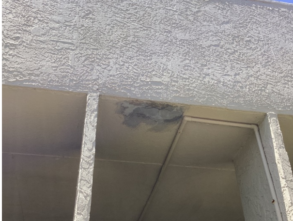
Elevated concrete – concrete patches evident
