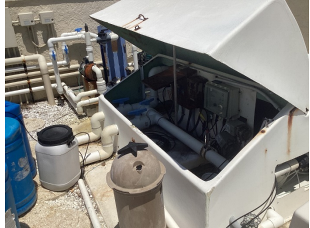
Pool mechanical equipment – overviews
