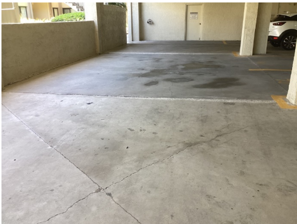
On grade concrete – cracks evident
