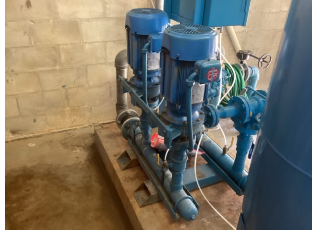
Domestic water pumps
