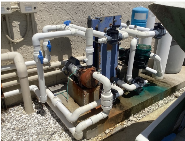
Pool mechanical equipment – overviews
