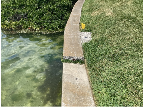
Cracks in the concrete cap evident
