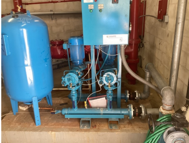
Domestic water pumps
