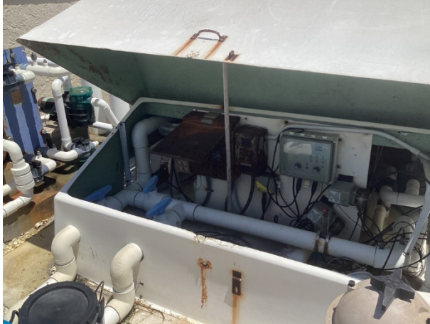
Pool mechanical equipment – overviews
