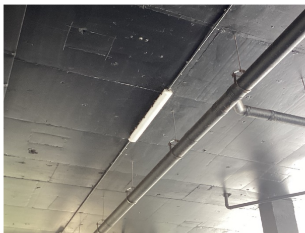
Garage light fixtures
