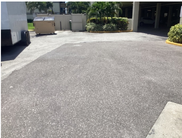
Asphalt pavement – previous patch repairs evident
