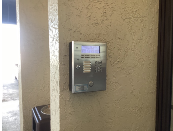
Intercom panel - typical
