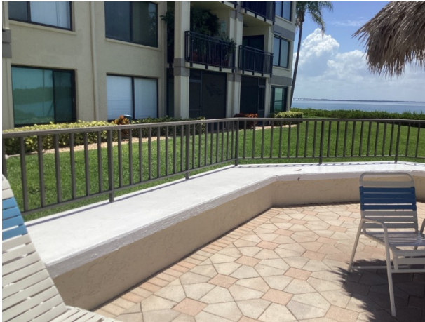
Pool fences - overview
