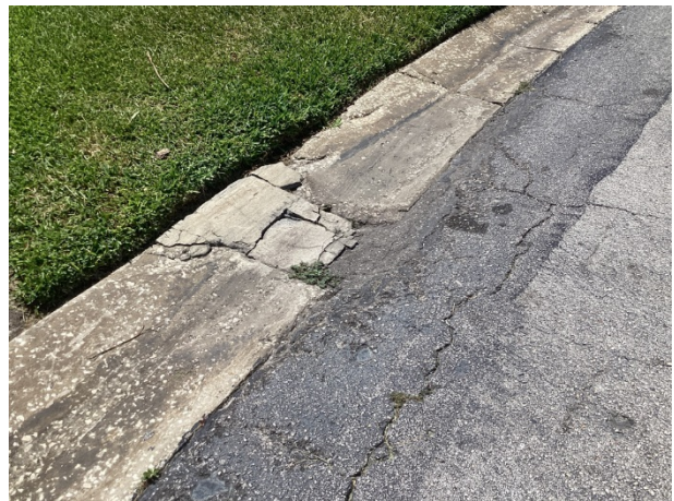
Asphalt pavement – cracks evident
