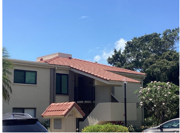
Concrete tile roofs – villas configuration
