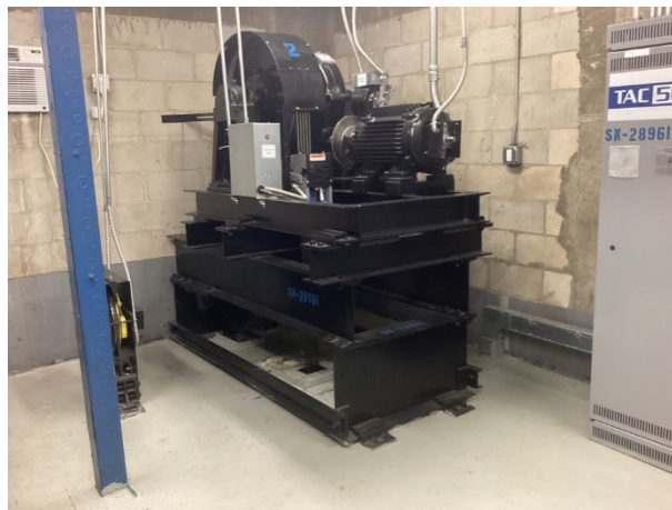
Elevator equipment - hoists
