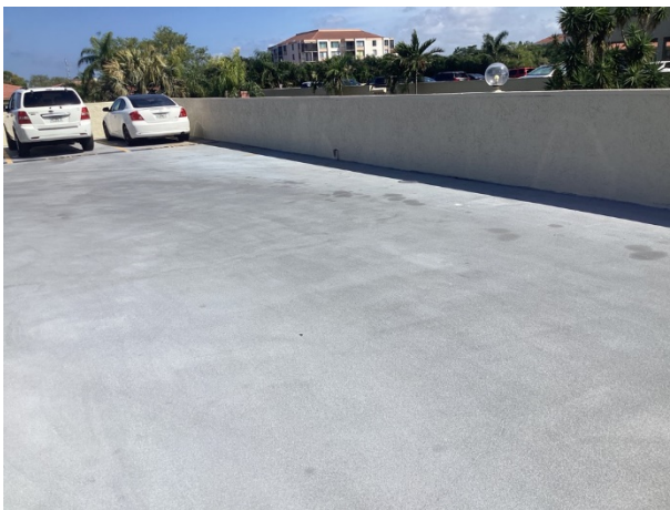
Traffic coating – deterioration evident
