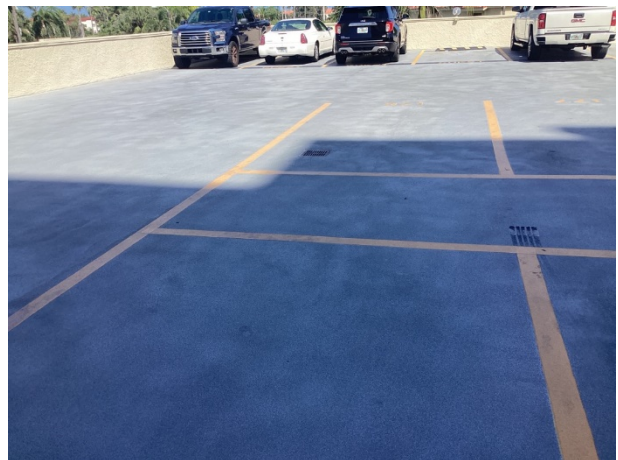
Traffic coating – deterioration evident
