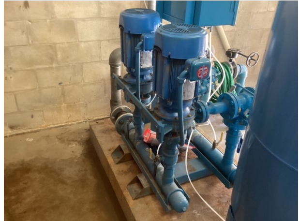
Domestic water pumps
