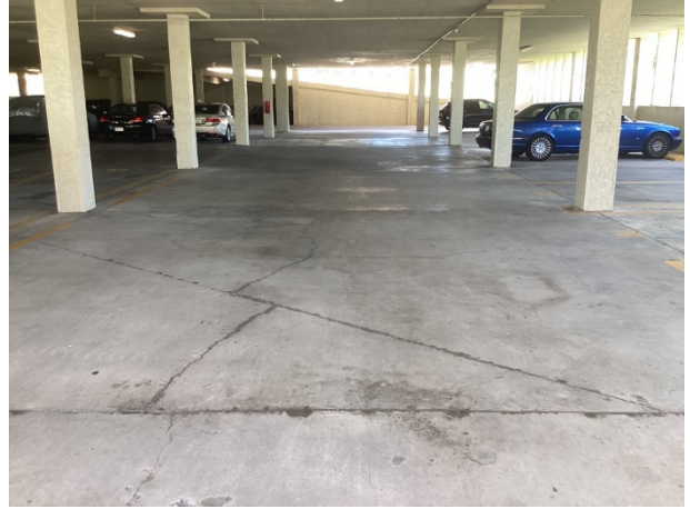
On grade concrete – cracks evident
