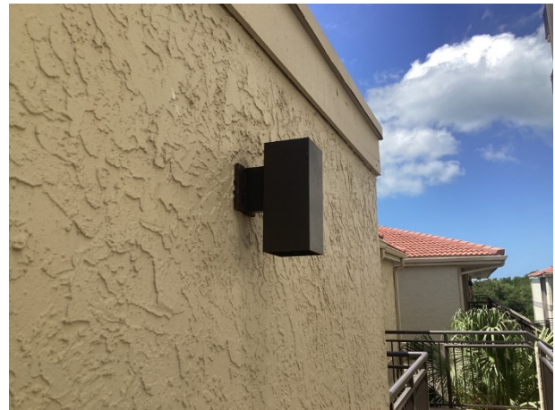
Light fixtures – globe fixture
