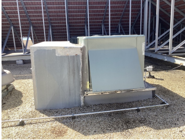
Roof top unit
