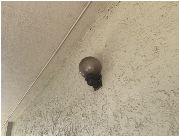
Light fixtures – globe fixture
