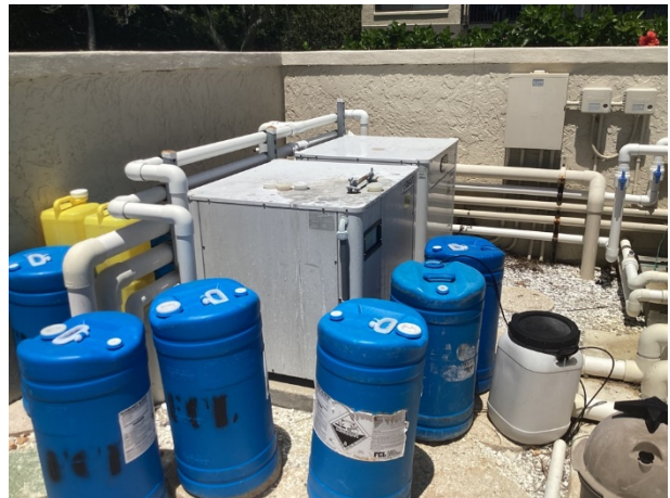
Pool mechanical equipment – geothermal heaters
