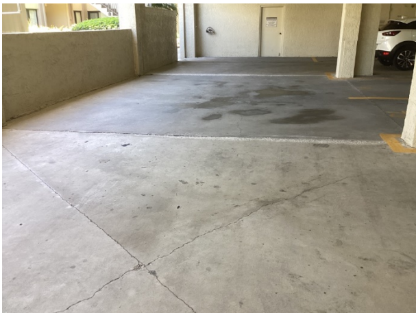
On grade concrete – cracks evident
