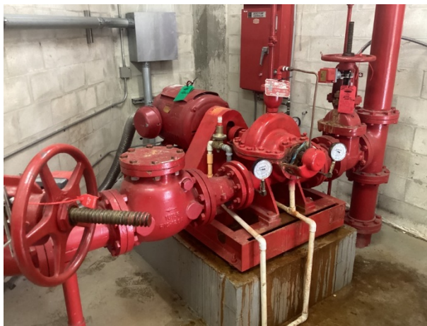
Fire pump - overview
