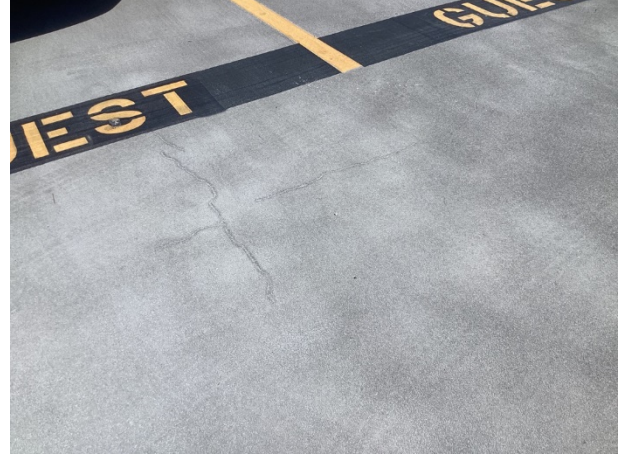
Elevated concrete – cracks evident
