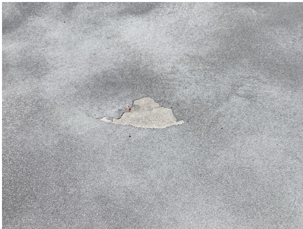
Traffic coating – deterioration evident
