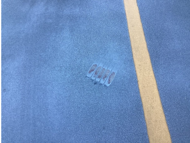
Traffic coating – deterioration evident
