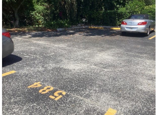
Asphalt pavement – deterioration of the seal coat application evident
