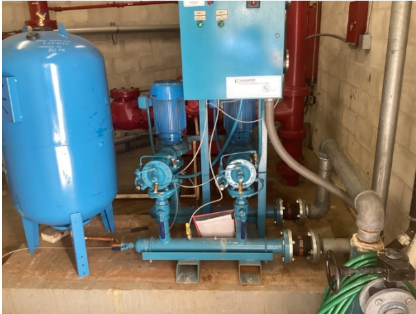
Domestic water pumps
