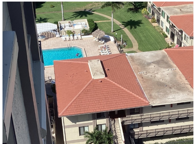
Concrete tile roofs – villas configuration
