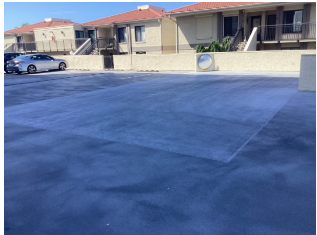
Traffic coating – deterioration evident
