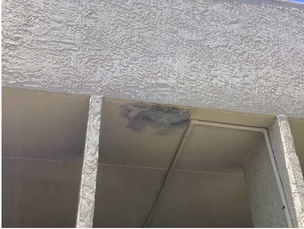
Elevated concrete – concrete patches evident
