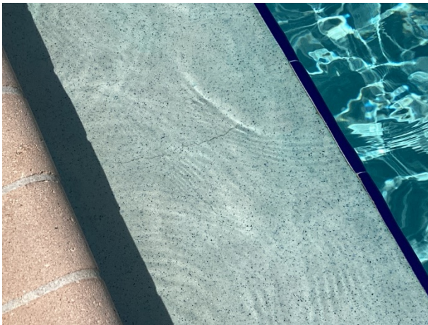
Pool finishes – cracks evident
