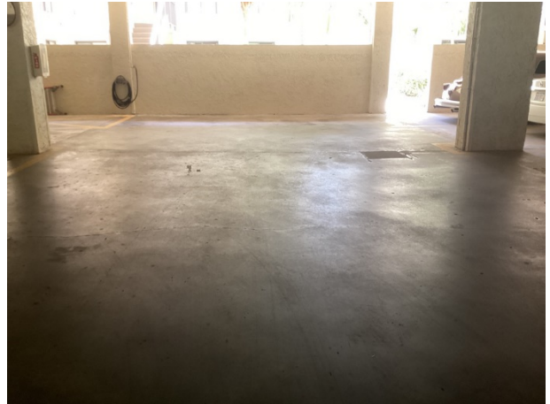
On grade concrete – cracks evident
