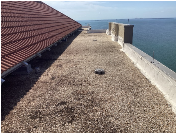
Built-up roof – granular loss evident
