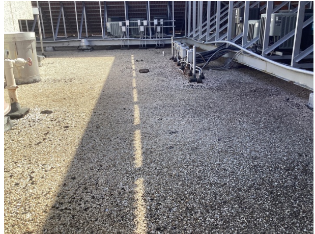
Built-up roof – granular loss evident
