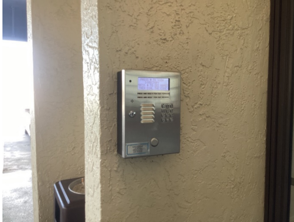
Intercom panel - typical
