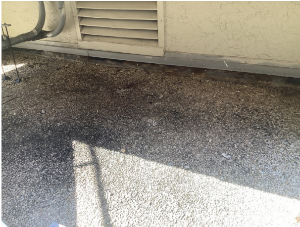
Built-up roof – granular loss evident
