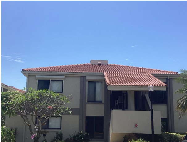
Concrete tile roofs – villas configuration
