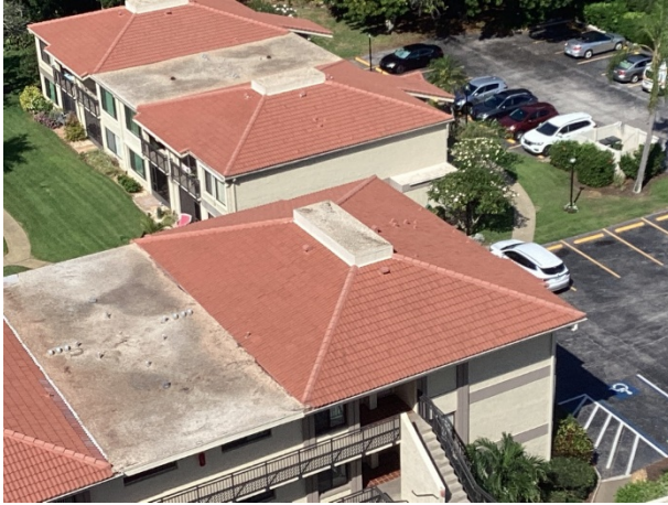
Concrete tile roofs – villas configuration
