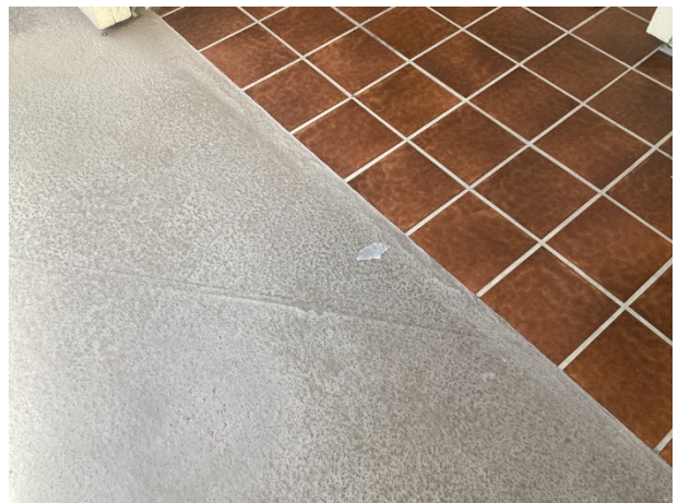
Breezeways – deterioration of the waterproof coating application evident
