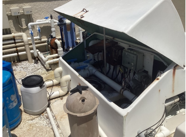
Pool mechanical equipment – overviews
