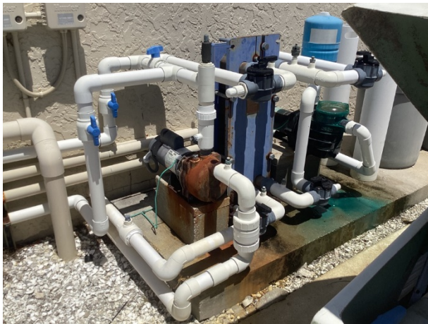
Pool mechanical equipment – overviews
