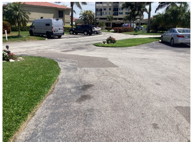
Asphalt pavement – deterioration of the seal coat application as well as cracks evident
