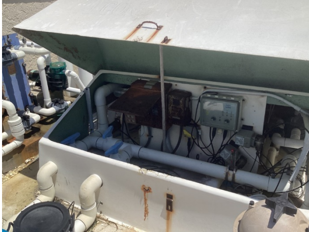
Pool mechanical equipment – overviews
