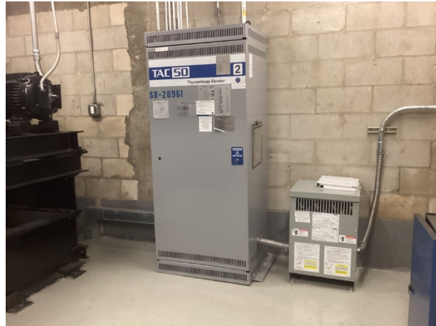
Elevator equipment – control panel
