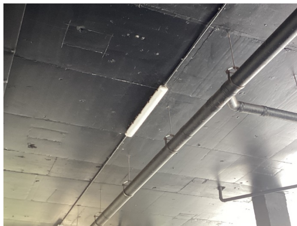
Garage light fixtures
