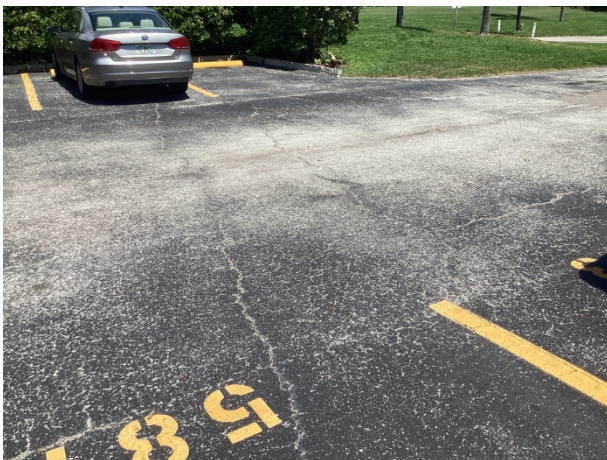
Asphalt pavement – deterioration of the seal coat application as well as cracks evident
