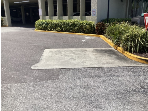
Asphalt pavement – deterioration of the seal coat application as well as cracks evident
