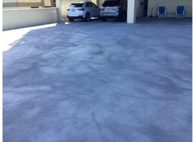
Traffic coating – deterioration evident
