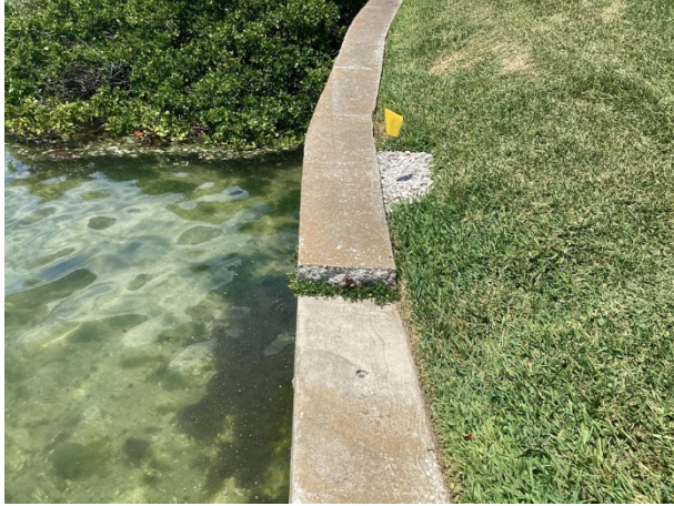
Cracks in the concrete cap evident
