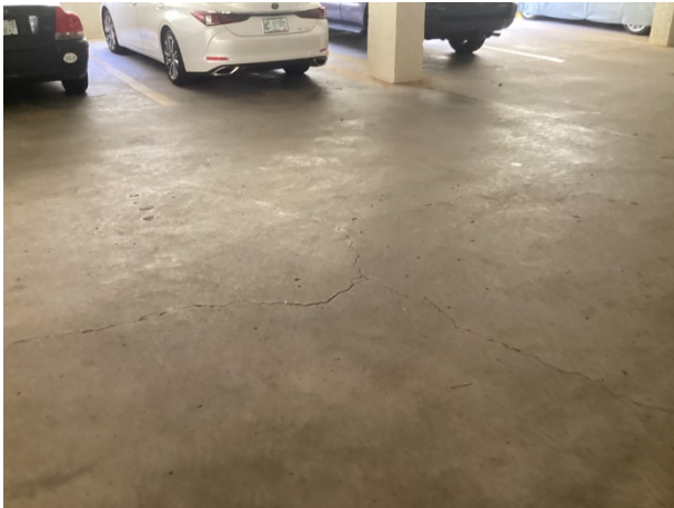
On grade concrete – cracks evident
