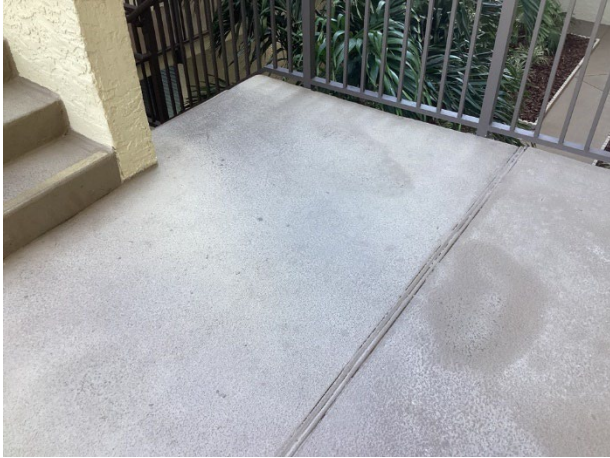
Breezeways – deterioration of the waterproof coating applications evident
