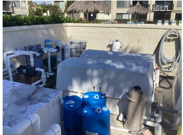
Pool mechanical equipment – overview
