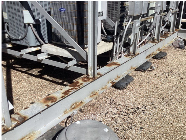
Steel structure – corrosion evident
