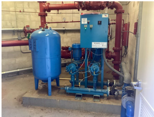
Domestic water pumps
