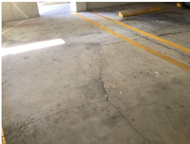
On-grade concrete – cracks evident
