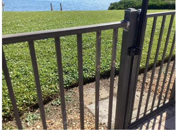
Fences – finish deterioration evident
