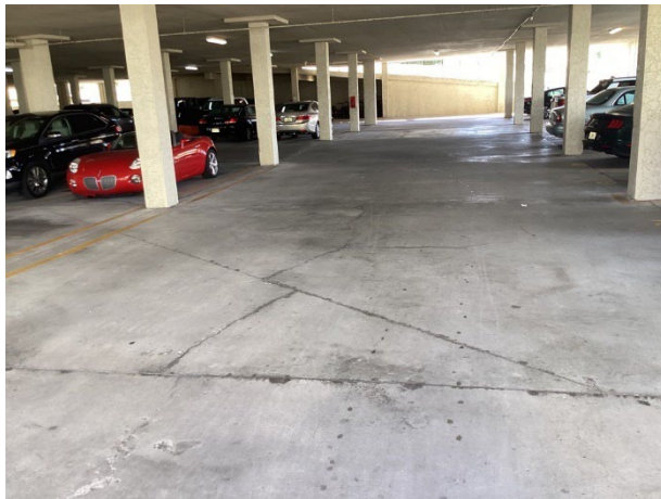
On-grade concrete – cracks evident
