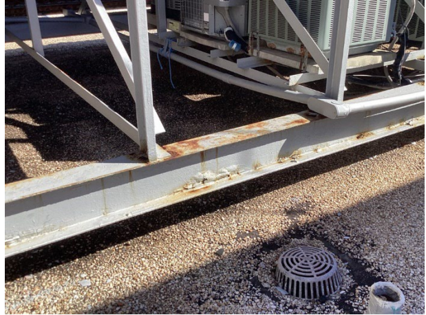
Steel structure – corrosion evident
