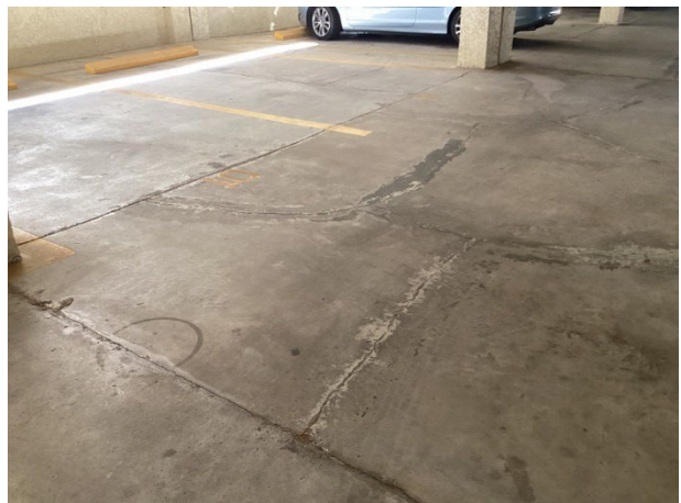
On-grade concrete – cracks evident
