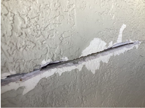
Paint finish applications – Tower – cracks evident
