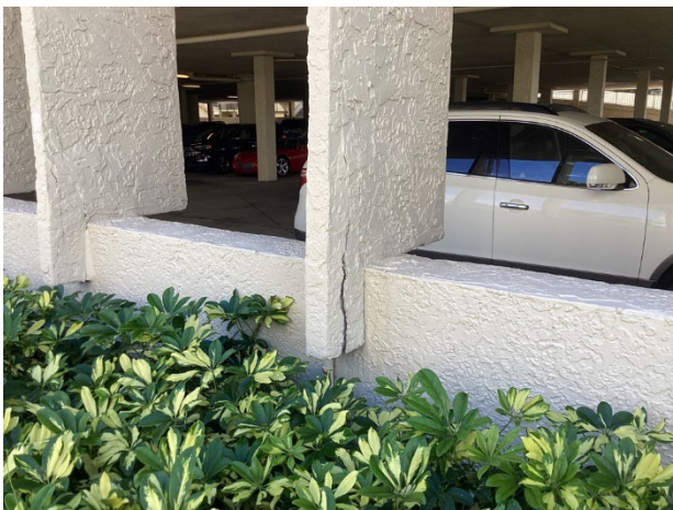
Paint finish applications – Garage – cracks evident
