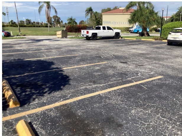
Asphalt pavement – alligator cracks evident
