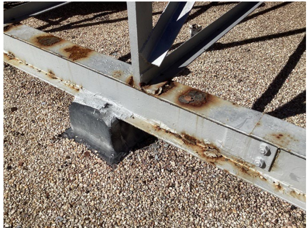
Steel structure – corrosion evident
