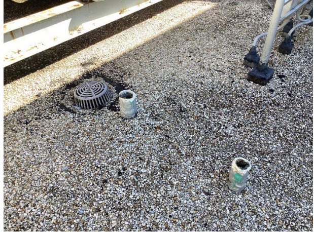
Built-up roof - granular loss evident
