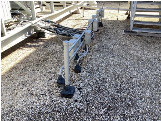
Built-up roof - granular loss evident
