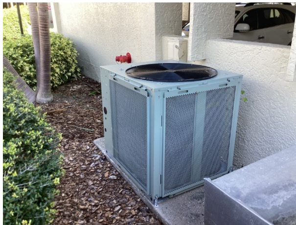
HVAC – split system
