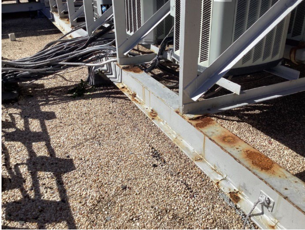
Steel structure – corrosion evident
