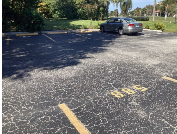
Asphalt pavement – alligator cracks evident
