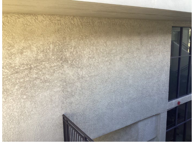
Paint finish applications – Tower – paint finish deterioration evident
