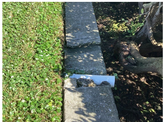
Seawall – cap deterioration evident
