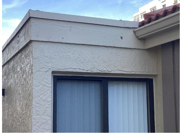
Paint finish applications – Villas – paint finish deterioration evident
