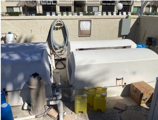
Pool mechanical equipment - overview
