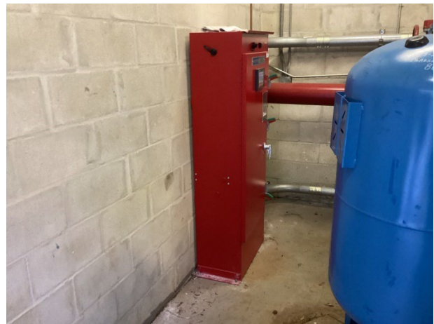
Fire suppression pump - controls
