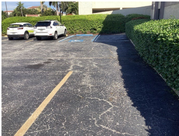
Asphalt pavement – alligator cracks evident
