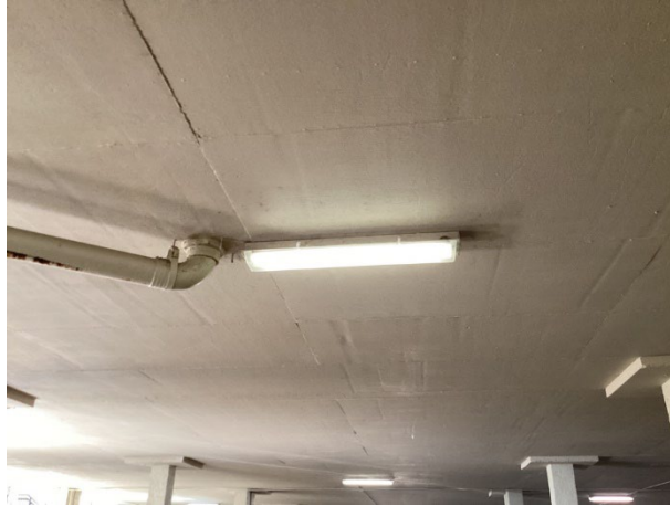
Light fixtures - overview
