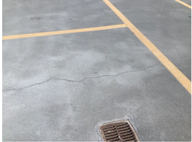
Elevated concrete – cracks evident
