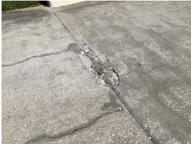
Elevated concrete – spalling evident
