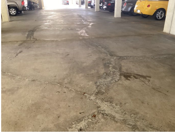
On-grade concrete – cracks evident
