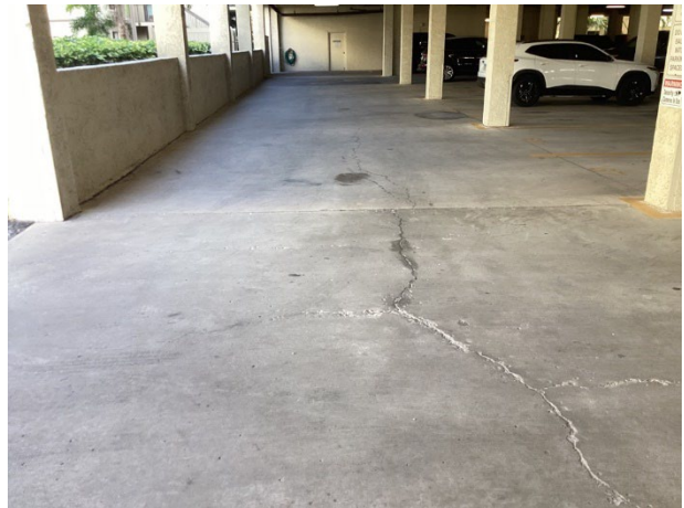
On-grade concrete – cracks evident
