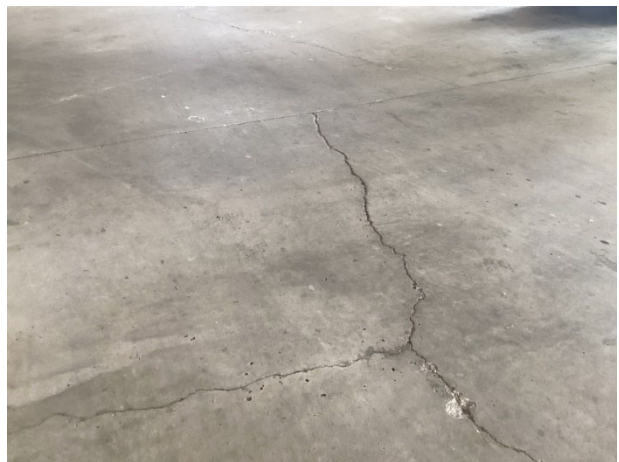
On-grade concrete – cracks evident
